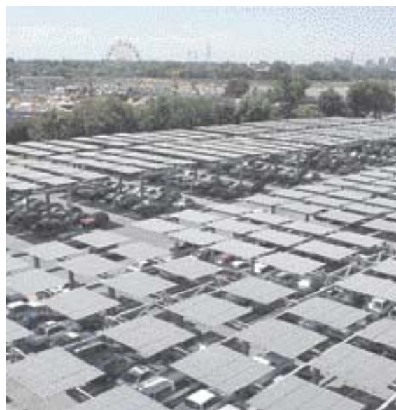
PV parking shelters in California, USA
