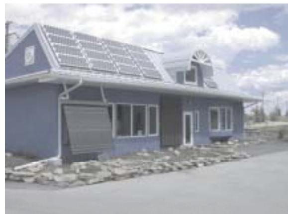
PV modules at the Airdie Environmental Centre, Canada
