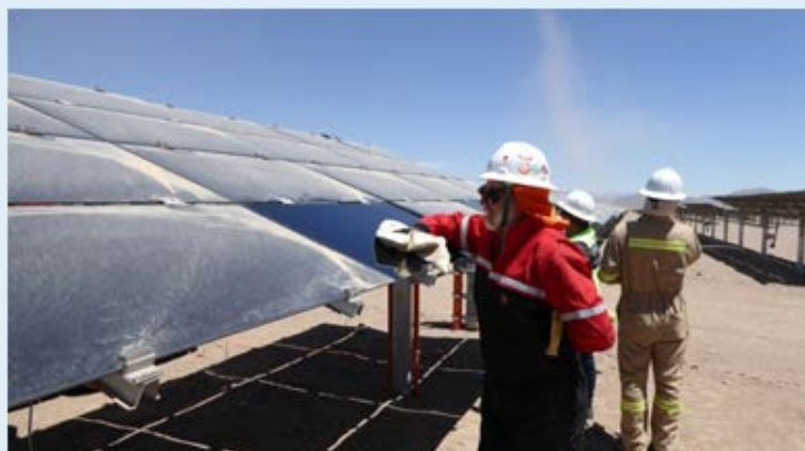
Fig.1: Example of extreme soiling on the 150 MWp PV power plant in Copiapo, Chile.
