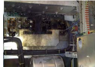
Fig. 7: Inverter failure due to an exploded insulated-gate bipolar transistor [4].
