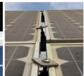
Fig. 20: Wrong combination of clamps and modules are used [3].
