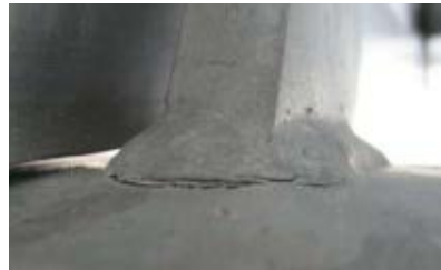
Fig. 13: Cracks due to mechanical stress [14].
