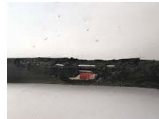
Fig. 28: Damage of cable due to rodent bite [22]
