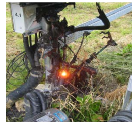
Fig. 4: A combiner box is destroyed due to fire [11]
