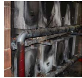
Fig. 3: Inverters are burned due to fire [8].
