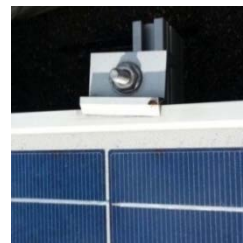
Fig. 19: Improperly installed end brackets [7].
