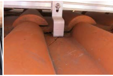
Fig. 18: Roof shingle has contact to roof tile [16].
