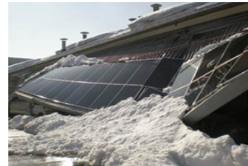
Fig. 14: Structural subsidence due to snow load [15].
