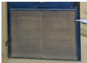
Fig. 6: A soiled air filter causes overheating 2 [3].
