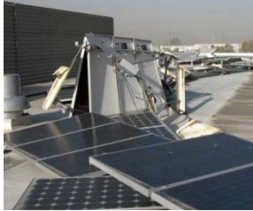
Fig. 9: Destroyed system after high wind load [18].
