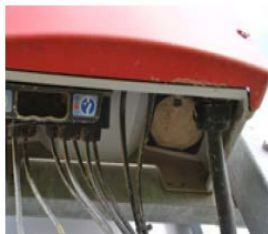
Fig. 5: A soiled air filter causes overheating 1 [3].
