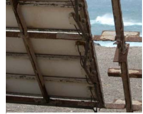
Fig. 11: Corrosion due to salt water [17].
