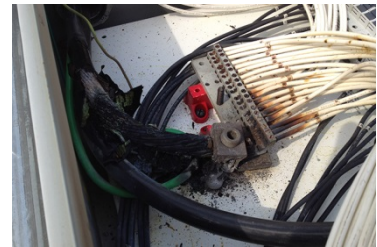
Fig. 26: Improper wire torquing causes a fire [10].
