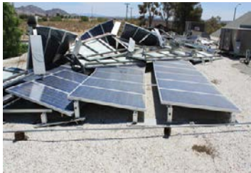
Fig. 12: Mounting system collapsed due to high wind load [13].
