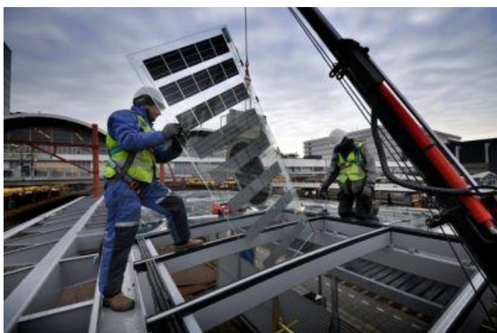
Figure 2-2: Solar panels are installed at Utrecht central station. (Source: www.duurzaammbbo.nl )
