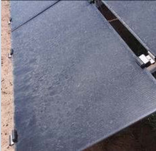
Dust accumulation on the PV panel
