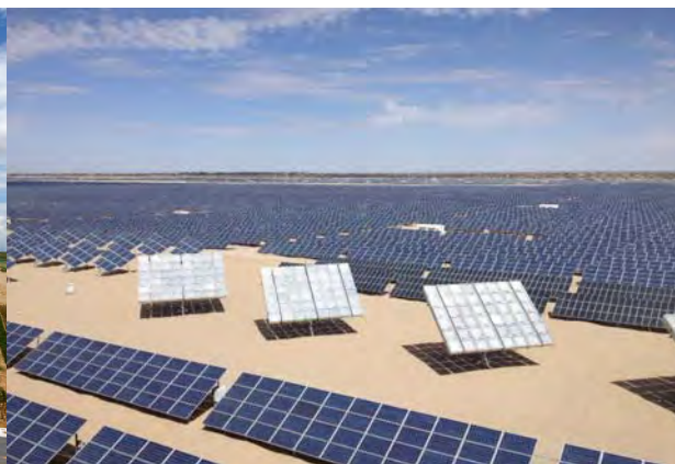
Fig. 1.1-4 The second largest PV power plant in Germud, Qinghai, 500 MW
