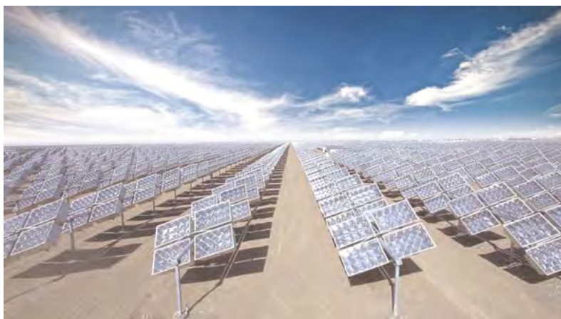
Fig. 4.1-7 A 50 MWp Suncore CPV system at Golmud, Qinghai Province, China [Courtesy of Suncore ]
