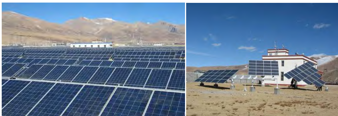
Fig. 1.1-1 100kW PV Power Plant at Yangbajing, Tibet
