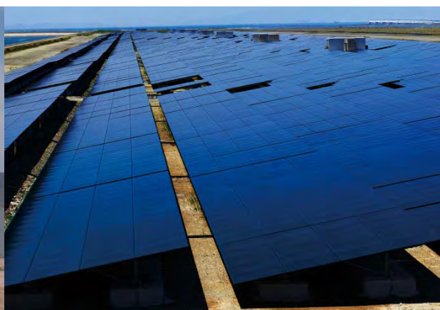
Fig. B.1-10 Osaka, Japan (12 MW, CIS) (courtesy of Solar Frontier K.K.)
