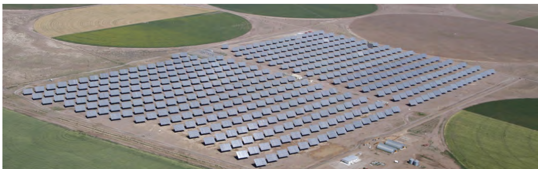
Fig. 4.1-4 A 30 MWp Arzon CPV system at Alamosa, CO, USA [Courtesy of Arzon Solar ]
