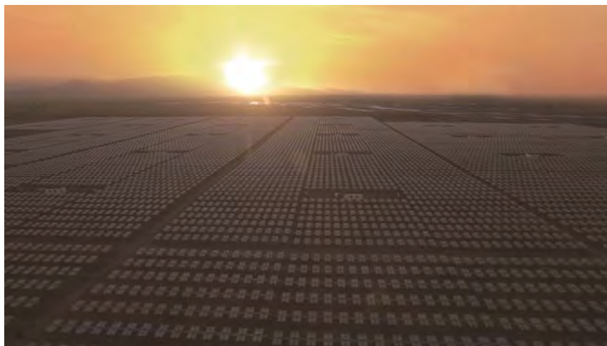
Fig. 6.1-9 Part of a 60 MWp CPV system at Golmud, Qinghai Province (Photo courtesy Suncore Corp)
