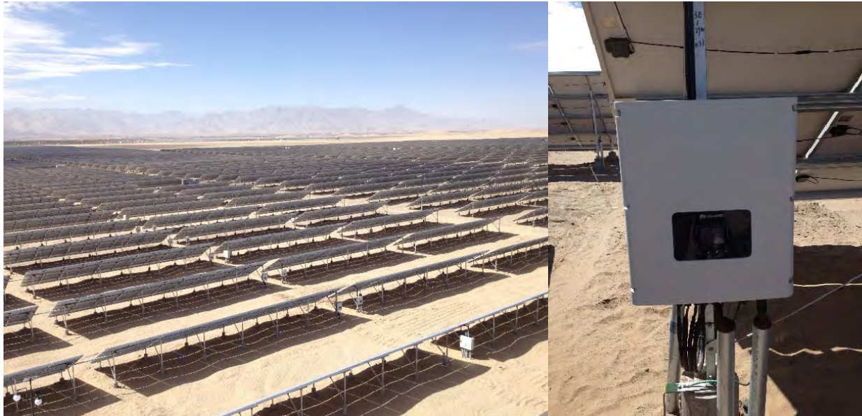
Fig. 1.1-24 PV power plant with string inverters (Total capacity of the plant is 500 MW, of which 200 MW with string inverters)
