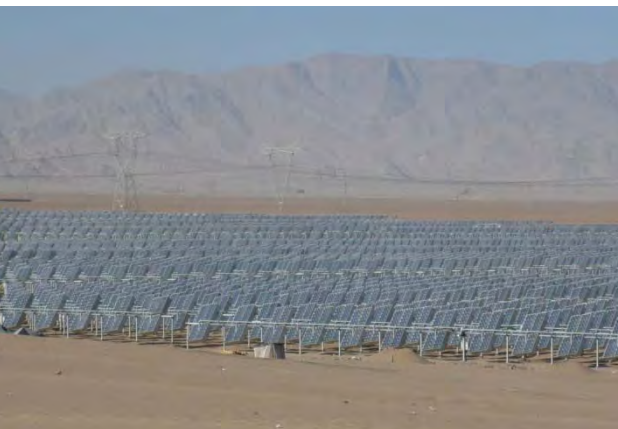
Fig. B.1-12 60MW HCPV in Qinghai, China
