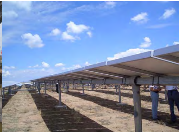
Fig 1.1-10 Horizontal E-W Sun-Tracking Systems with Bearing-Free Turning Axis at APS Test Field
