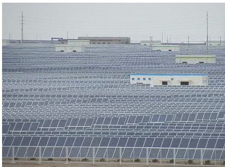
Fig 6.1-6 Part of a 1 GWp VLS-PV plant at Dunhuang, Gansu Province, China (Photographed by DF in July 2012)
