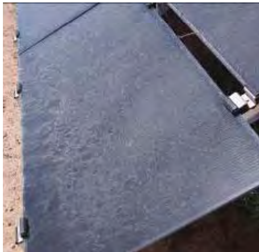
Dust accumulation on the PV panel
