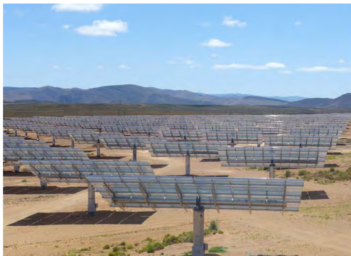
Fig. 4.1-6 A 44 MWp Soitec CPV system at Touwsrivier, South Africa [Courtesy of Soitec ]
