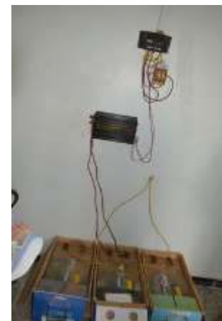
Figure 22: Poor installation of the installed PV system
