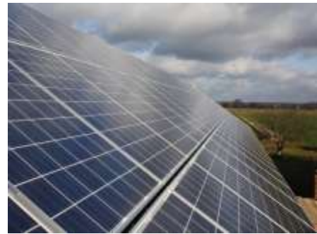
Figure 6: Crystalline Silicon PV array Source: phoma GbR
