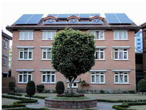
Rooftop solar array installed by Gham Power at Maiti Nepal.
