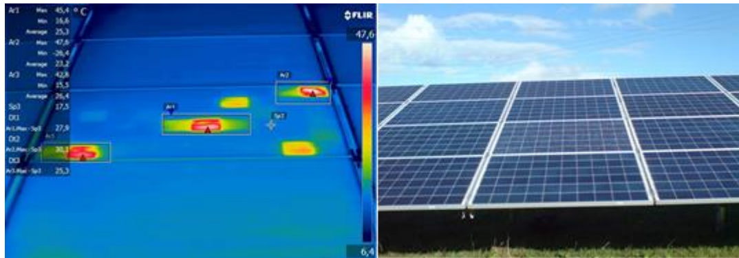
Figure 2-6: Breakage of front glass.
