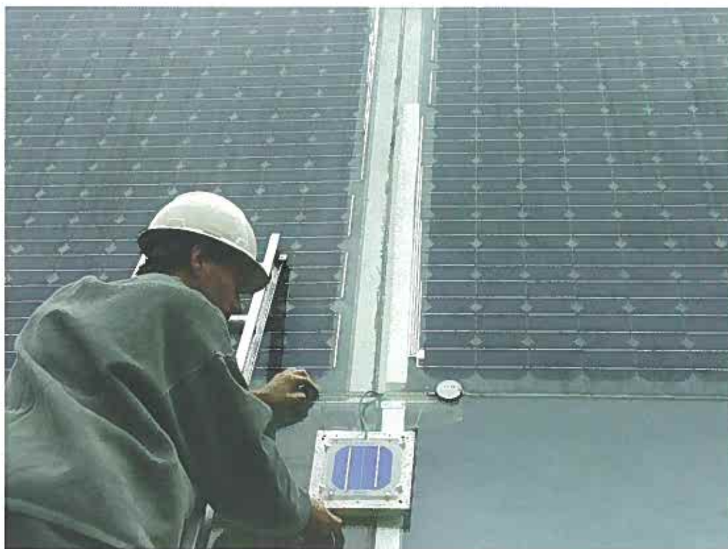
PV Thermal Facade experimental programme at IT Power (Task 7).
