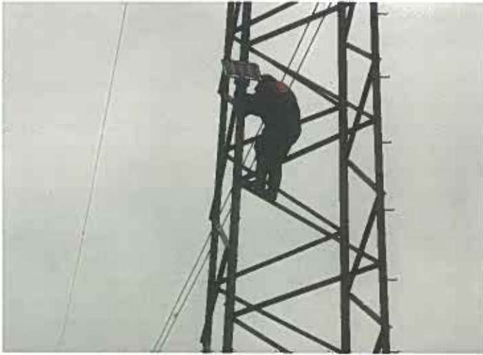
Installation of PV-module for cathodic corrosion protection of power pylons. There are approximately 50 000 pylons of this type in Sweden (Photo: Mårit Forssander, The Swedish Corrosion Institute 1998).
