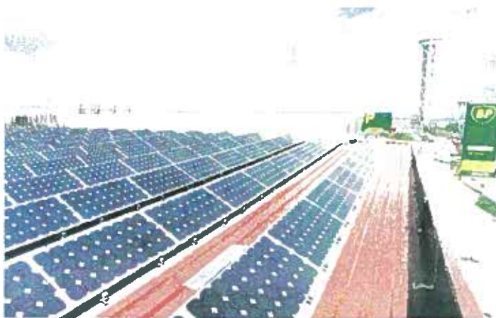
Fig. 2: BP "Sunflower" Project: 20,9 kWp grid-connected system (BP, Lisbon)
