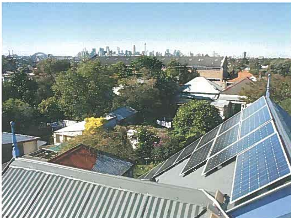
"A Pacific Solar 'Plug & Power TM' installation (photo courtesy of Pacific Solar)"
