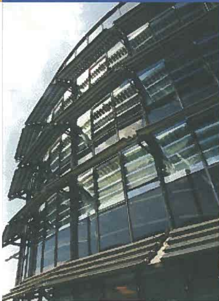
Figure 3: 20 kWp PV facade, office building of SBL, Linz (Colt)
