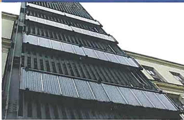
Building integrated 2 kW system at the University of Rome
