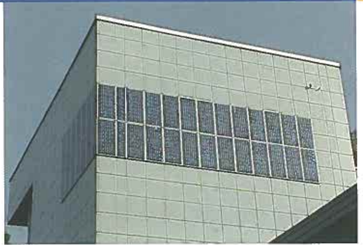
Grid connected 2,3 kW facade at a professional school in Trento
