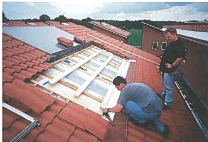
Fig. 1: One of 23 houses in the lagune project in Langedijk, wich form part of the 5 MWp City of the Sun. The houses have systems varying in size between 3 and 8 kWp, adding up to a total of 130 kWp. Because of smart project organisation and system design, system prices were achieved of less than 5 Euro per Wp (excl of VAT) (Copyright Novem - Hans Pattist)
