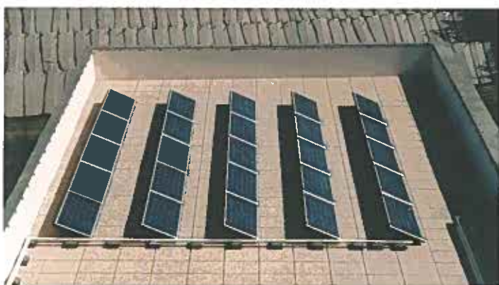
Fig. 1: 5 kWp AC-Module PV System (EDP, Faro)
