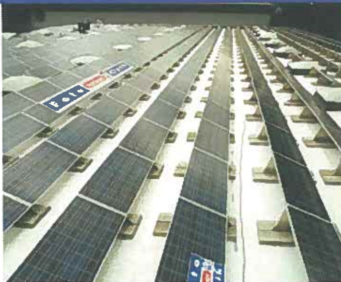
Figure 1: 75 kWp PV rooftop installation of Hartlauer company/Steyr (Electronic and photo stores)
