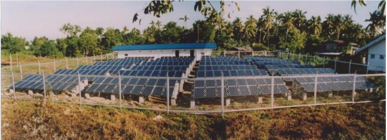
Isolated PV installation in the Philippines
