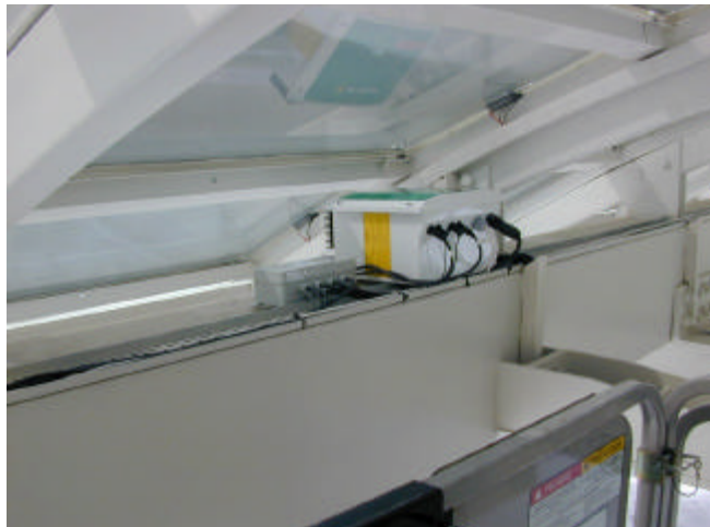
Photo 2. – PV modules electrical connections and support structure
