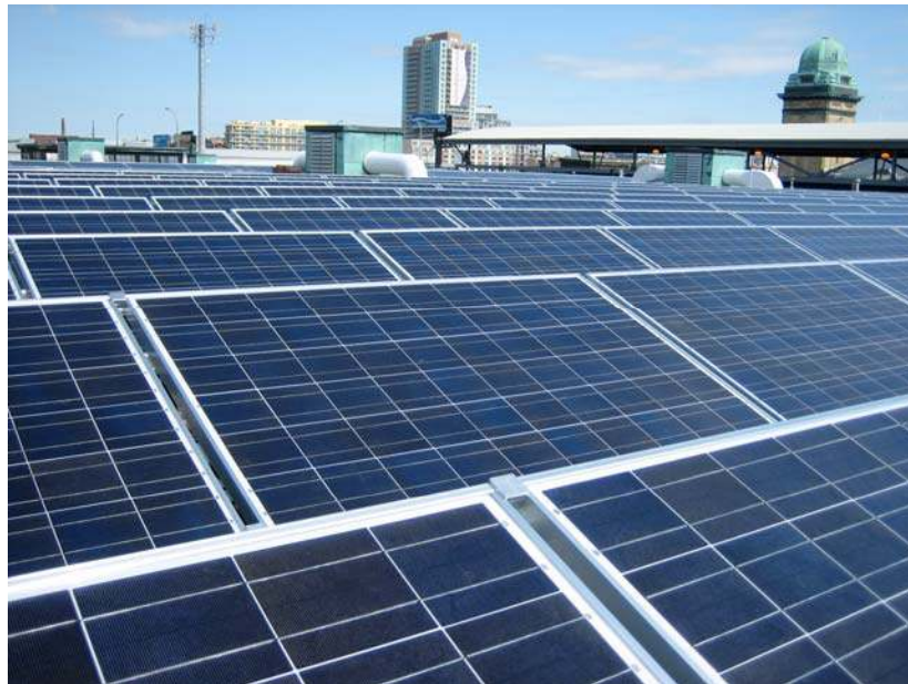
Fig. 1: 1100 kW PV roof-mounted installation at exhibition Place, Toronto, Ontario, Canada. (Photo credit Exhibition Place)
