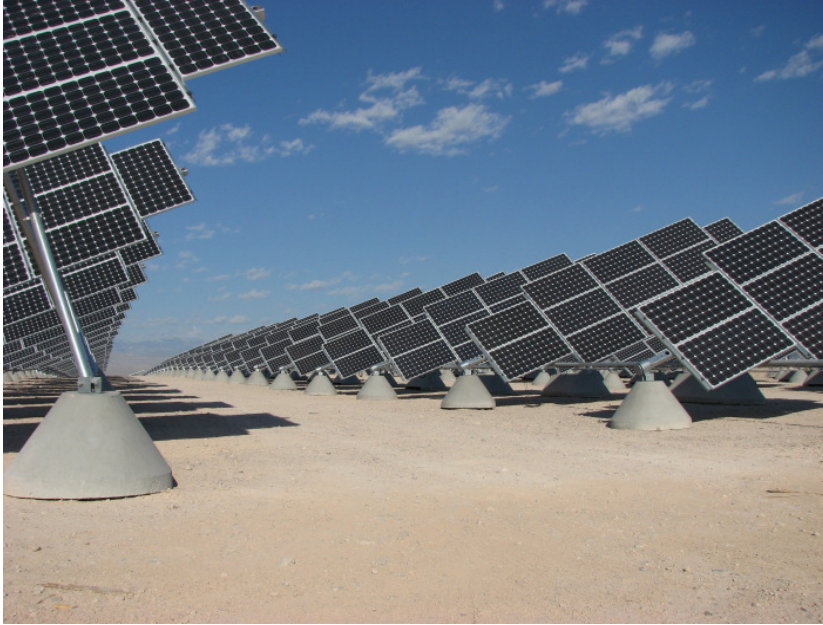
A 14,2 MW PV power plant at Nellis Air Force Base, Nevada.
