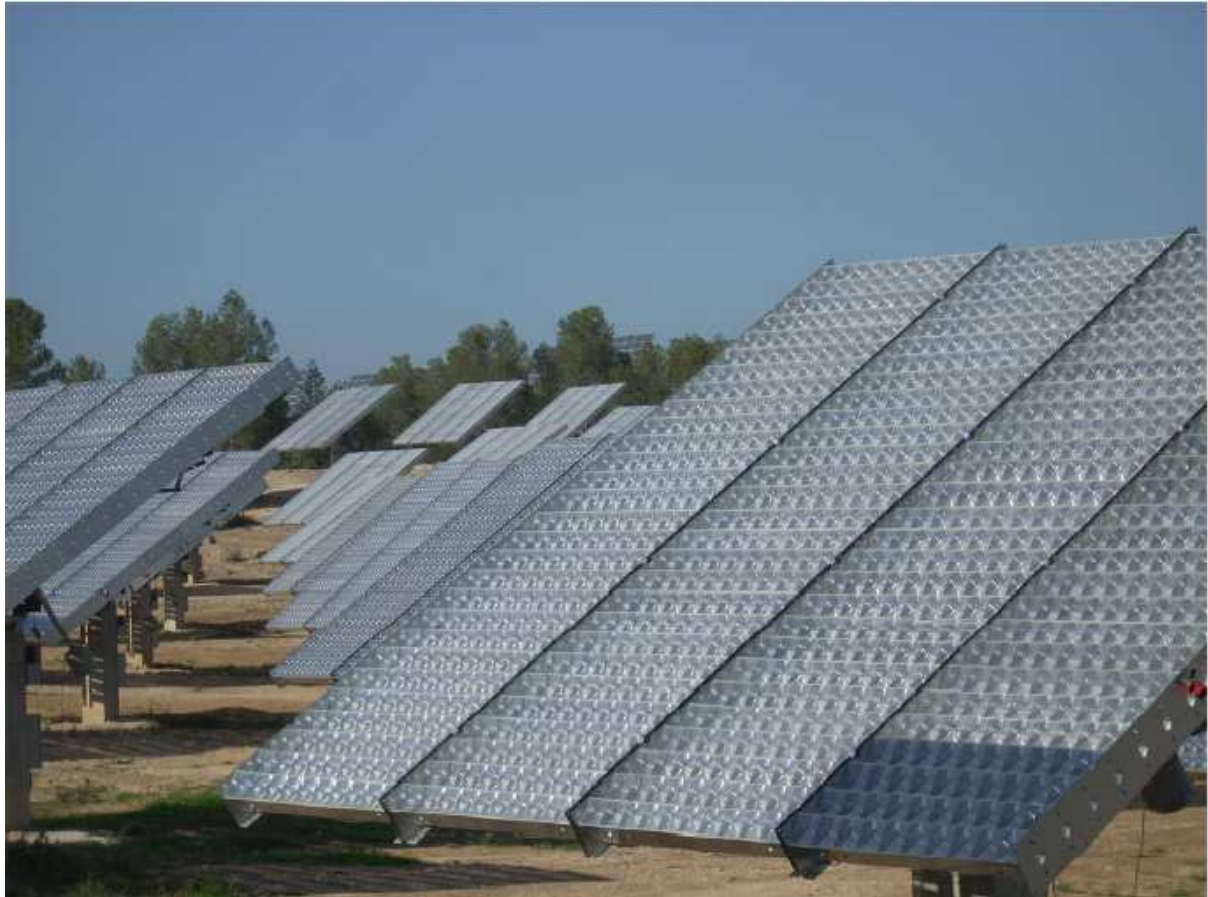
Figure 19 High concentration photovoltaic plant (800 kW) in Flix (Tarragona)
