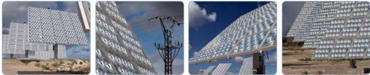
Figure 21 High Concentration PV plant (300 kW) installed in Almoguera for the Institute of Concentration Photovoltaic Systems (ISFOC)
