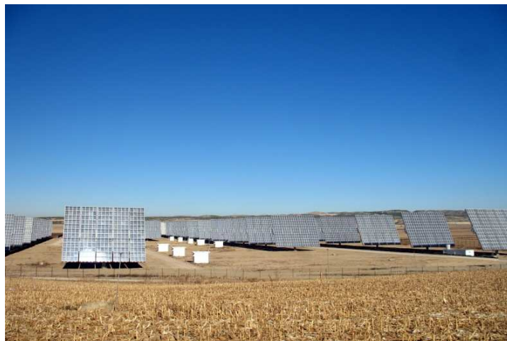
Figure 18 High Concentration PV plant (7.8 MW) installed in Villafranca (Navarra)
