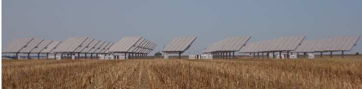
Figure 17 High Concentration PV plant (1.5 MW) installed in Écija (Sevilla), with 60 trackers
