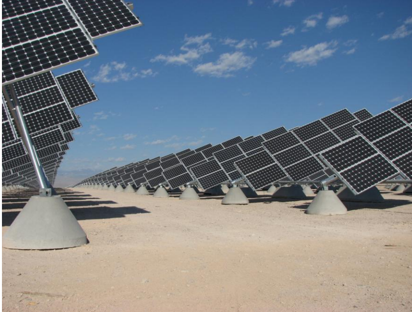
Figure 2: A 14,2-MW PV power plant at Nellis Air Force Base, Nevada.
