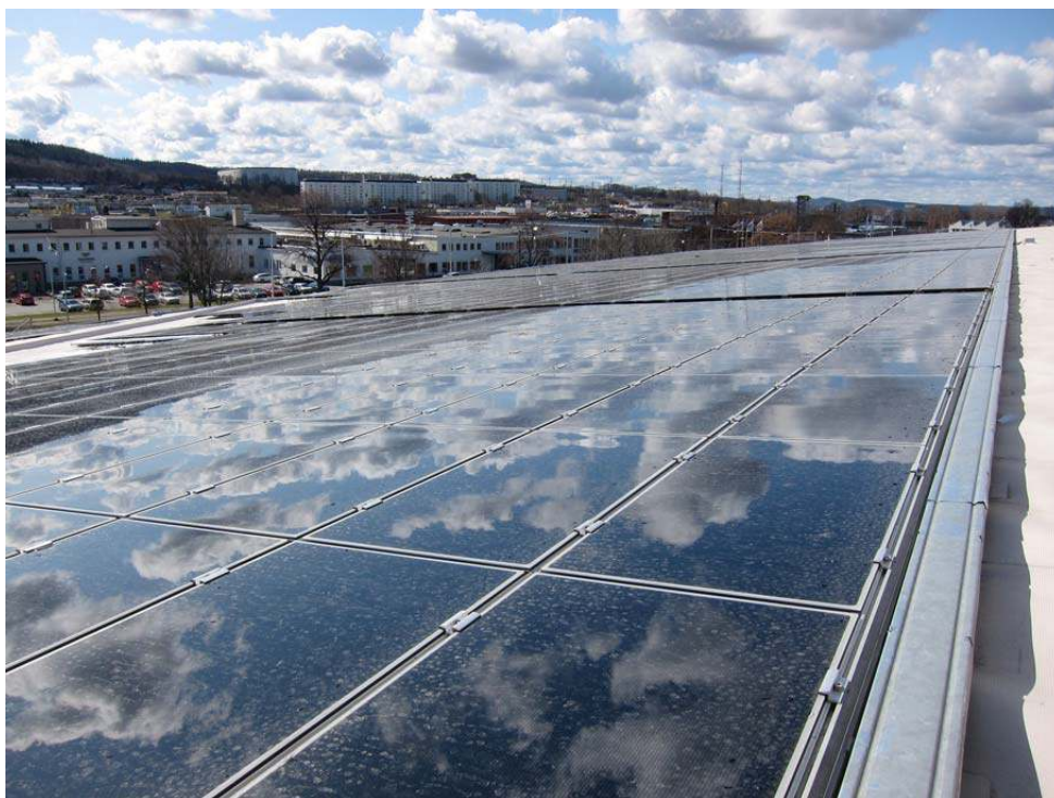
Figure 4: A thin film PV system installed at the roof top of the public bath Rosenlundsbadet, Jönköping (Courtesy Glacell)
