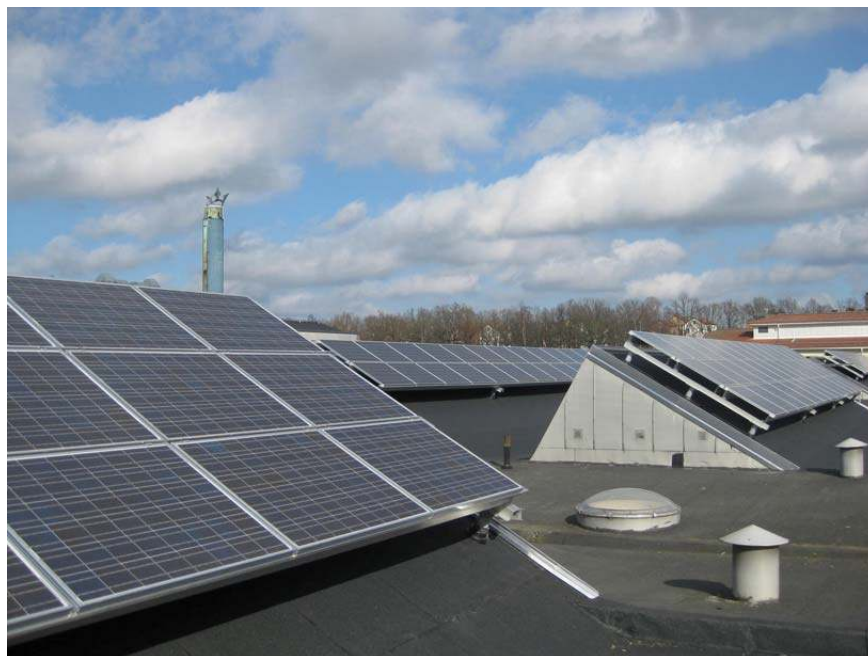
Figure 1: An example of a grid-connected roof top mounted PV system located at Kungsmadskolan, Växjö (Courtesy Mats Andersson)
