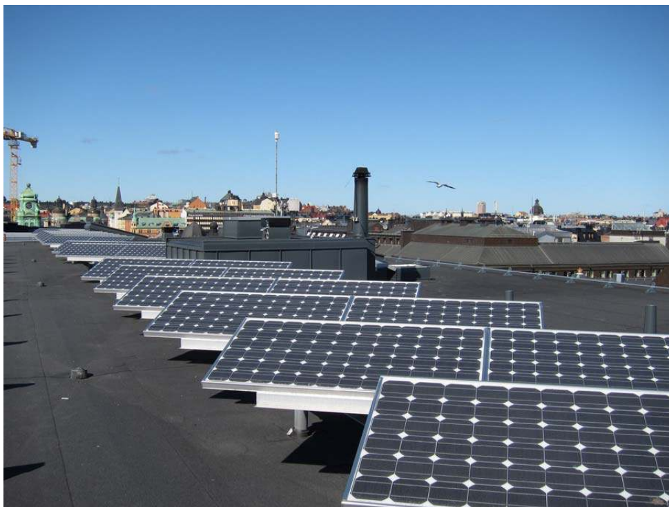
Figure 2: A roof top installation through the new investment subsidy at Pennfäktaren in central Stockholm (Courtesy Glacell)
