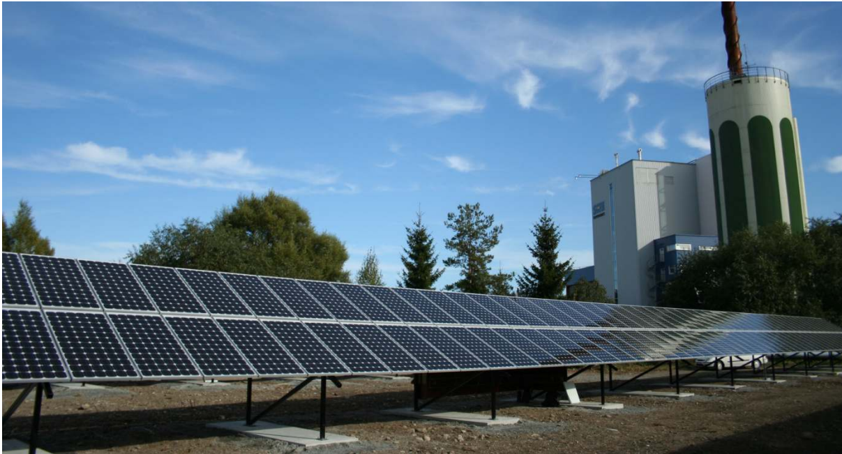
Figure 2: The second of the two systems that are covered by the FiT agreement in Sala-Heby. The system has a capacity of 78 kW. (Courtesy Solel i Sala & Heby ekonomiska förening and Hans Nyhlén)
