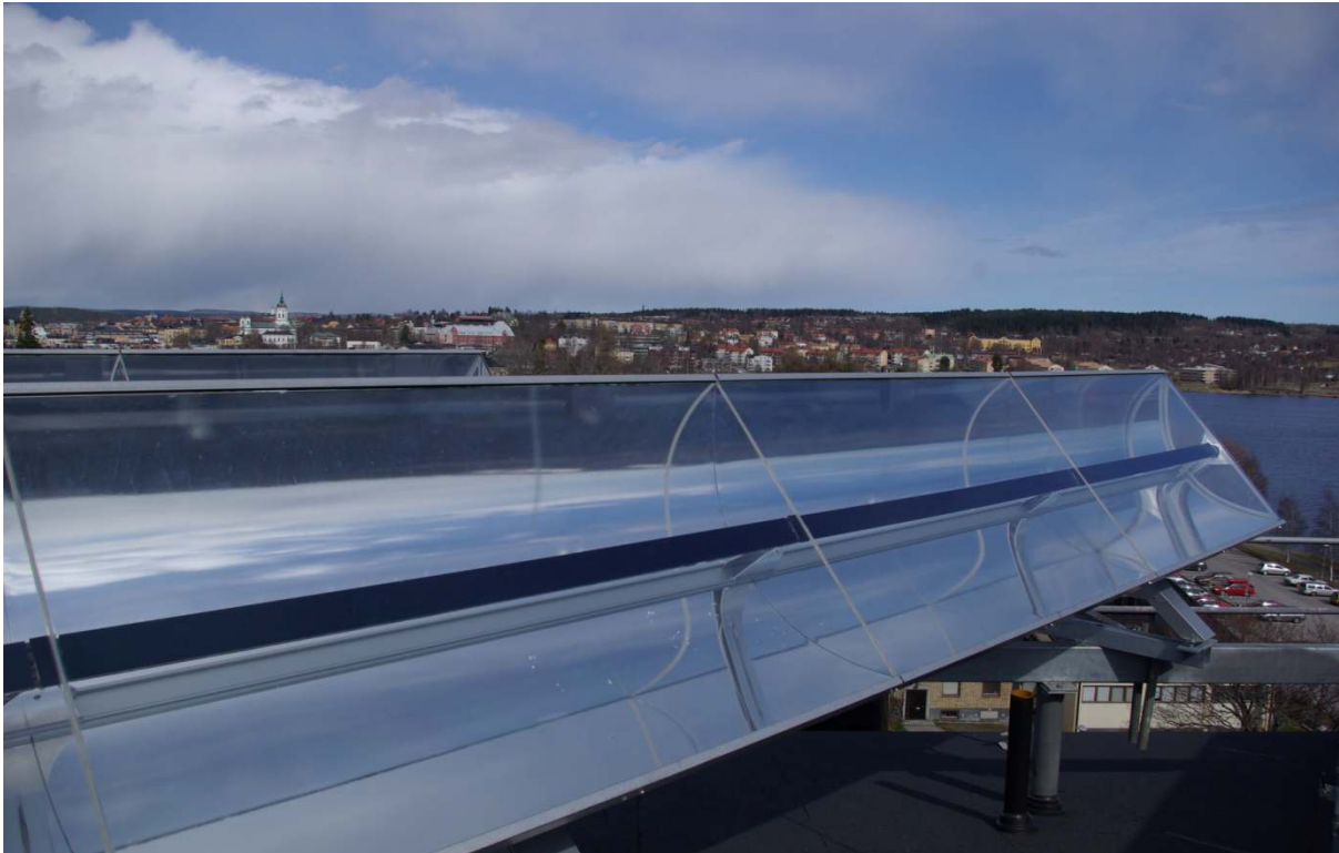
Figure 3: On the roof of the hospital in Härnösand stand solar panels that generate both power and heat simultaneously. (Courtesy Absolicon and Joakim Byström)
