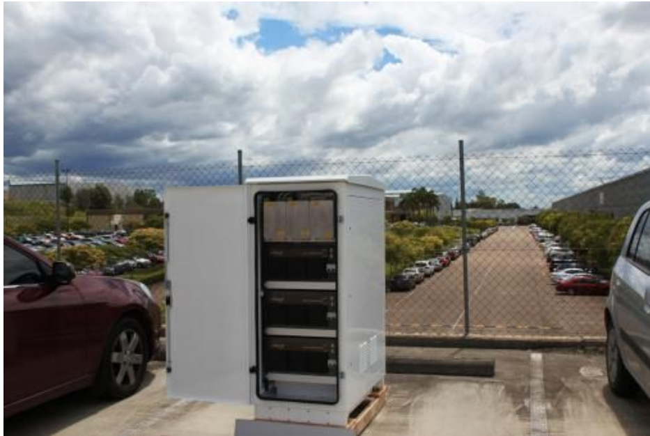
Figure 12: Three 20 kVA Statcoms arranged for 3 phase operation in a single rack mounting case
