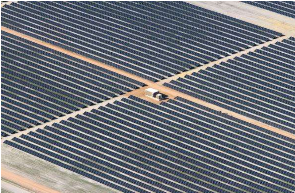
Figure 3: The 10 MW Greenough River PV Power Station, Western Australia (Photo: First Solar)
