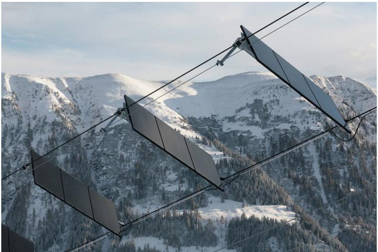
Picture 1 Solar Skilift Tenna, Switzerland
