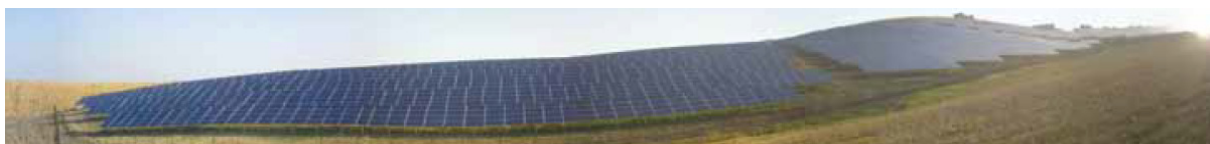
Figure 2 – 3,5 MW Montenero PV Plant at Campobasso (Photo: Hfv spa).
