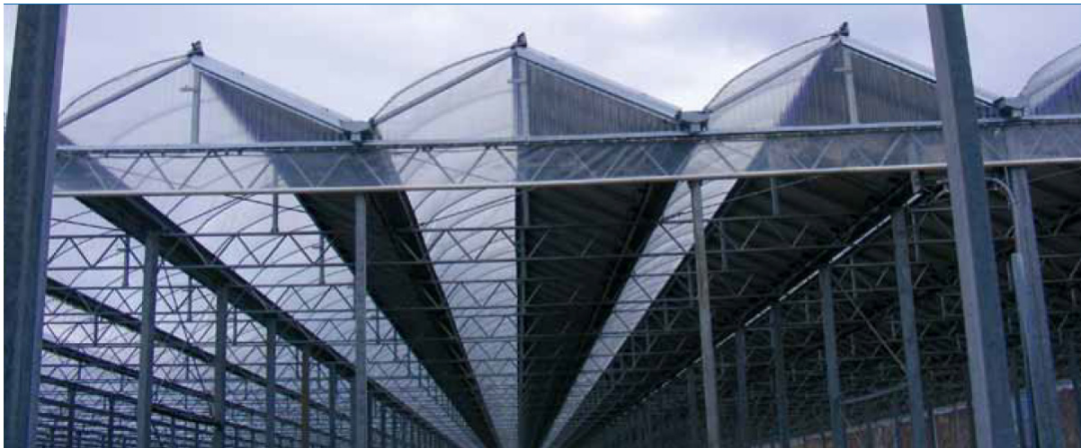
Figure 1 – 3,0 MW Orsomarso PV Plant on a greenhouse at Cosenza (Photo: Hfv spa).
