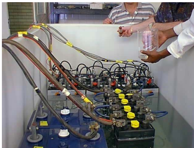
Figure 2: Acceptance testing of batteries
