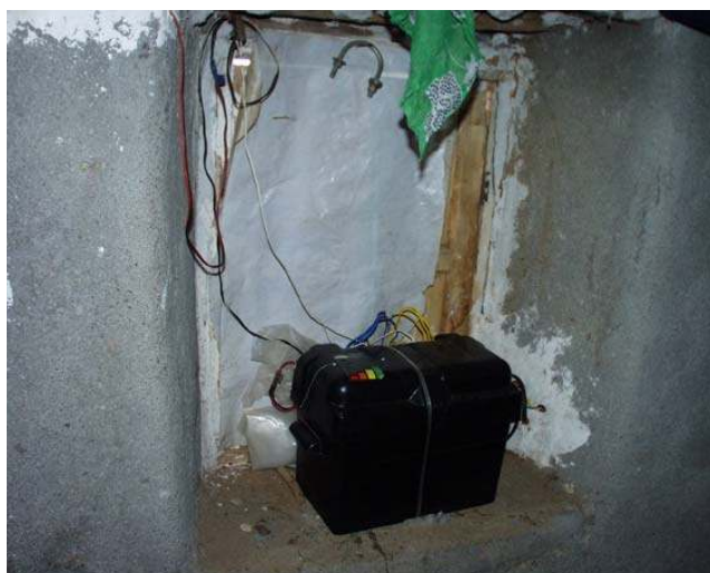
Figure 3: Poor system installation
