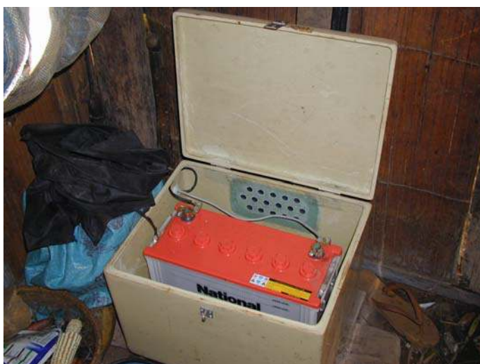
Figure 4: Example of a safely installed battery
