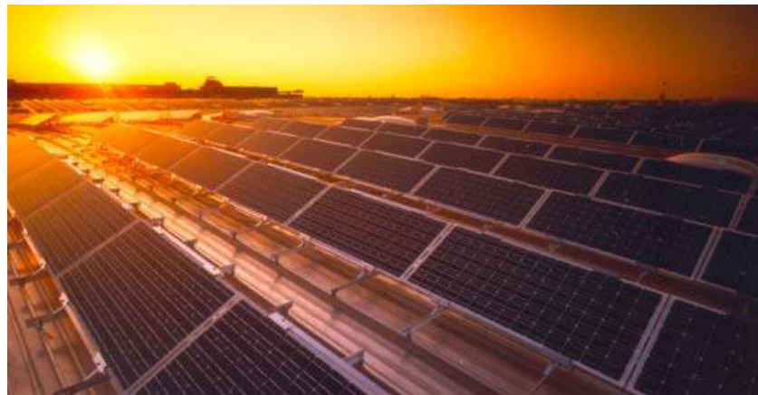
Fig. 1.18: General overview of the Munich Trade Fair Centre roof integrated PV system (Courtesy of Solarenergieförderverein Bayern e.V.).
