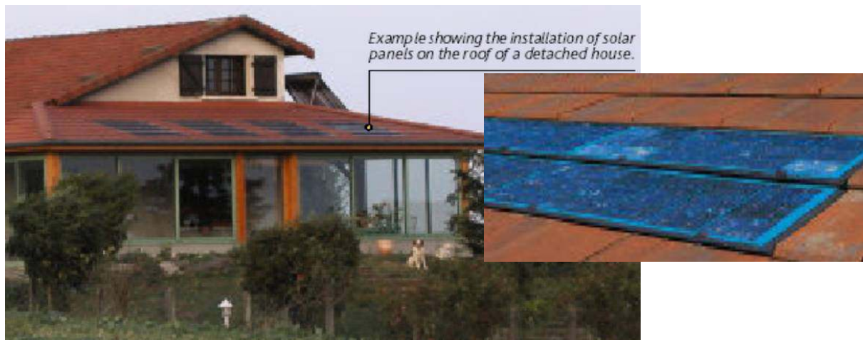
Fig. 2.4: Picture of the F1 PV system near Lyon and its PV roofing tiles.
