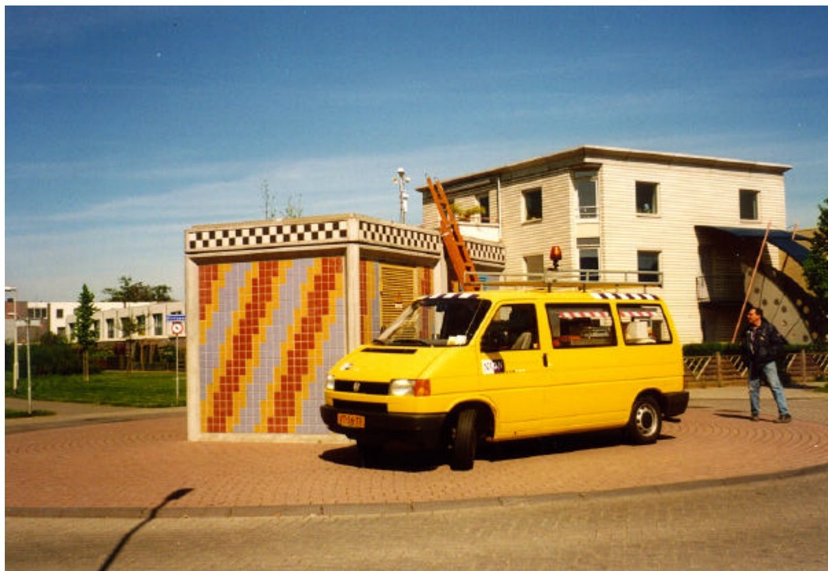
Figure 3.5 Power distribution cabinet with power transformer and low voltage busbar.
