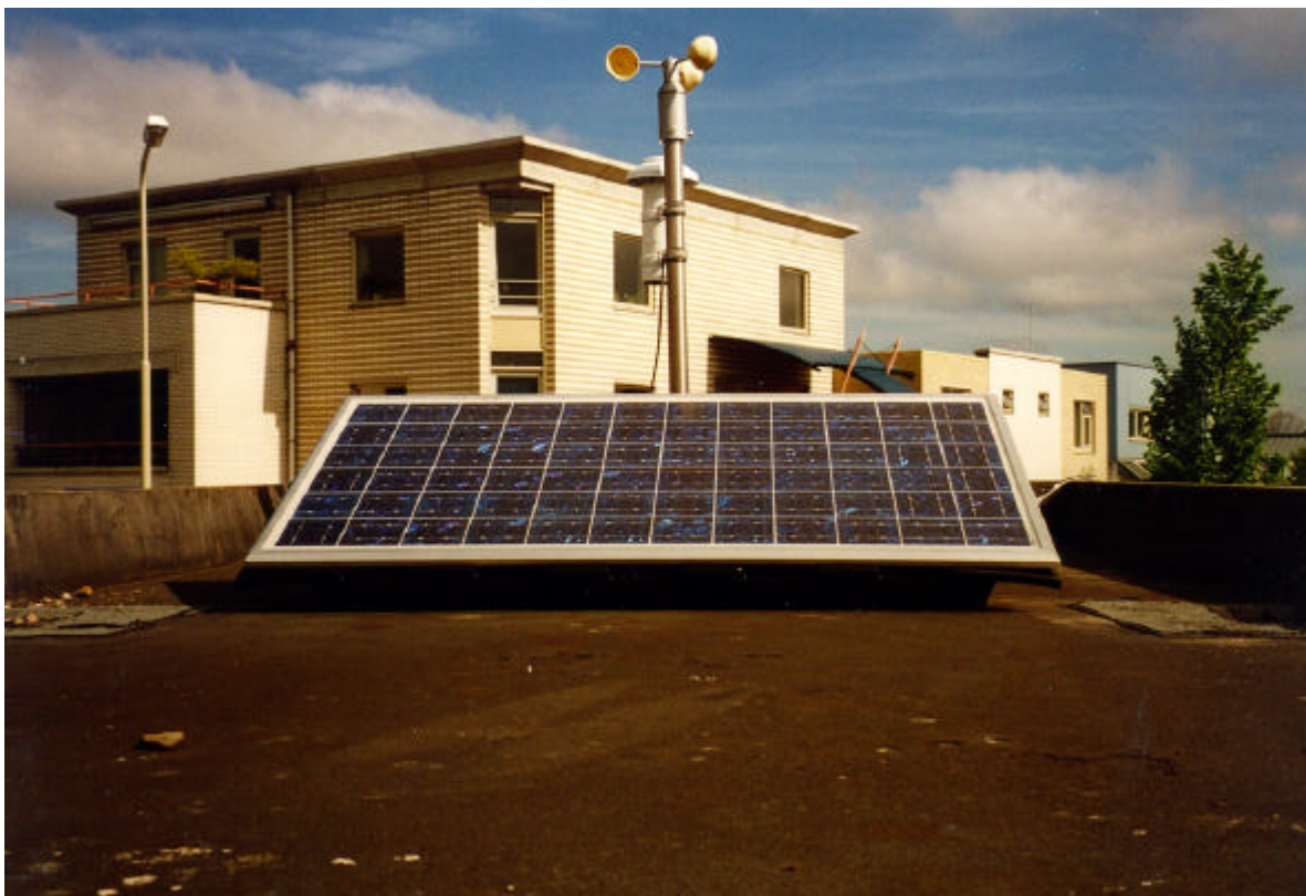
Figure 4.3 PV-panel, wind and temperature sensors on the roof of the transformer cabinet.
