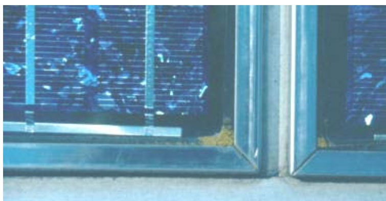
Fig. 11: Modules at Fraunhofer ISE after 11 years of operation.
