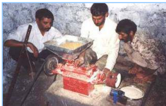
Small scale hydropower provides basic services such as rice hulling for food security
