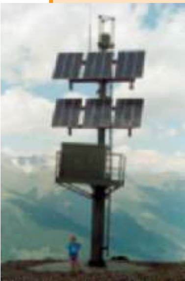
Security light for an alpine airport near St. Moritz, Switzerland
