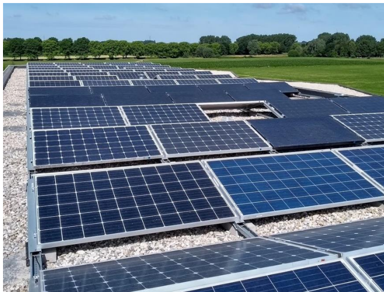
Waasland Cohousing Community (Sint-Niklaas, Belgium). For this PV installation, 226 second-life PV modules were combined with 5 new PV modules. (Photo credit: CIRCUSOL)
