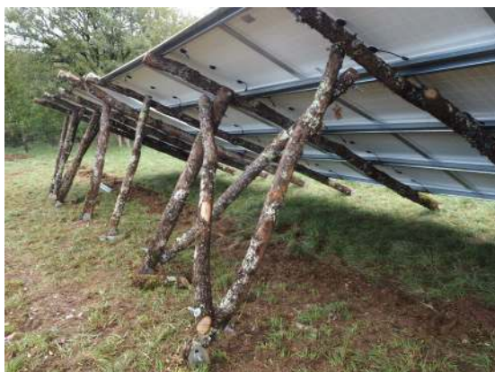
Figure 1: Simple logs used as supports for a 250 kW system in Carayac, France - Image credits Céléwatt
