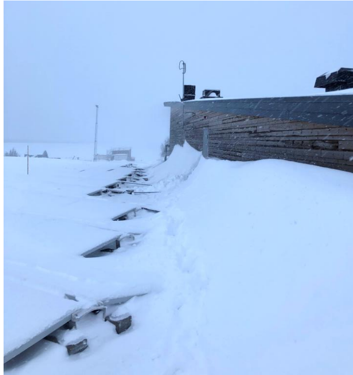
Rooftop PV [Piteå, SE]
