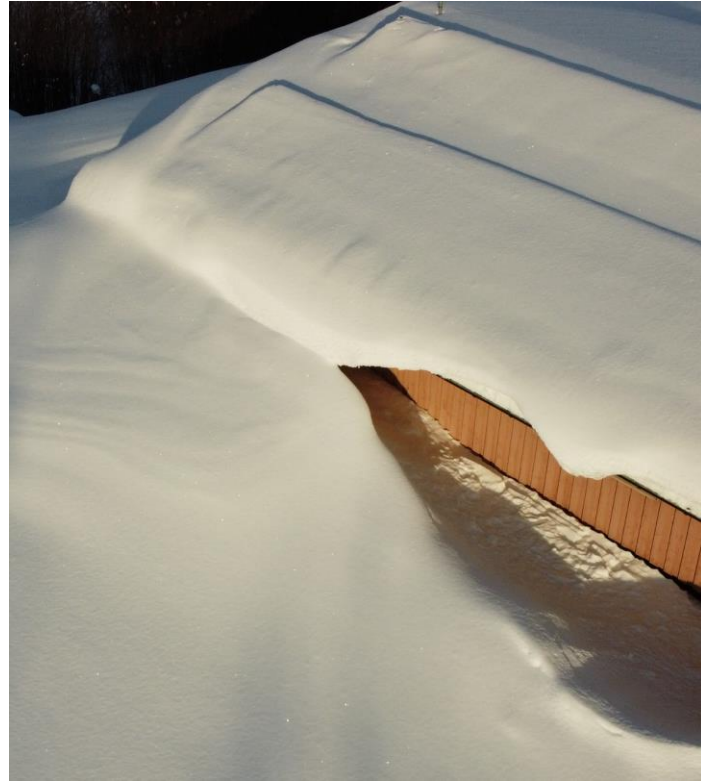
Snow covered rooftop PV [Piteå, SE]
