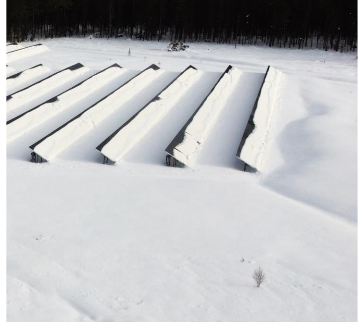
PV installation where snow cannot shed [Östersund, SE]
