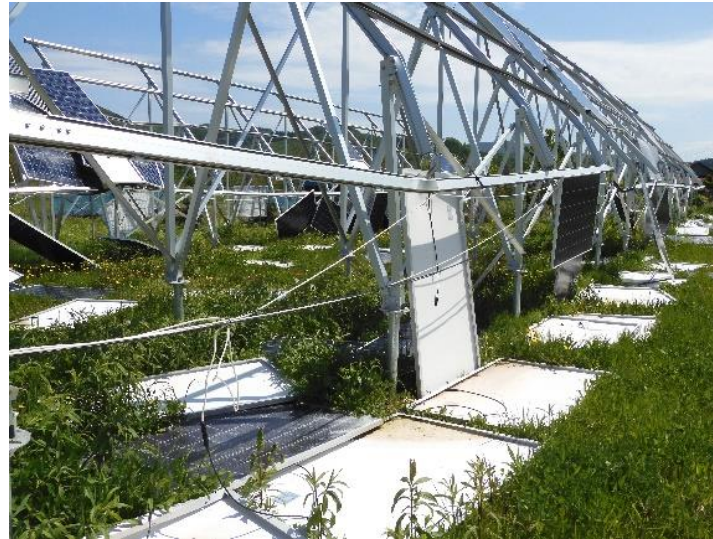
Deformation (tilting) of the horizontal rail
