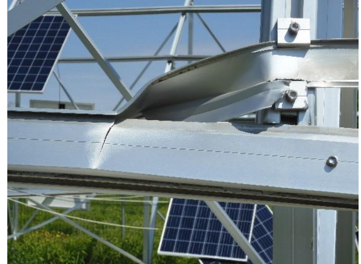
Tear at the joint of the horizontal rail
