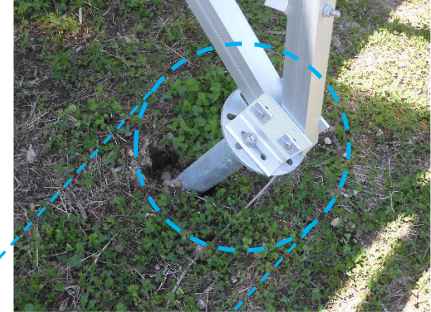
Tilt of the piles
