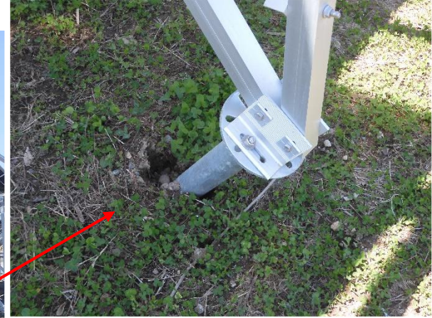
Tilting of the piles was also observed.
