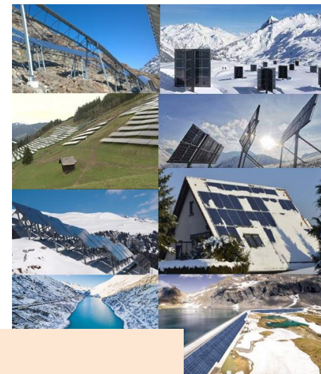
Installation in the alpine
