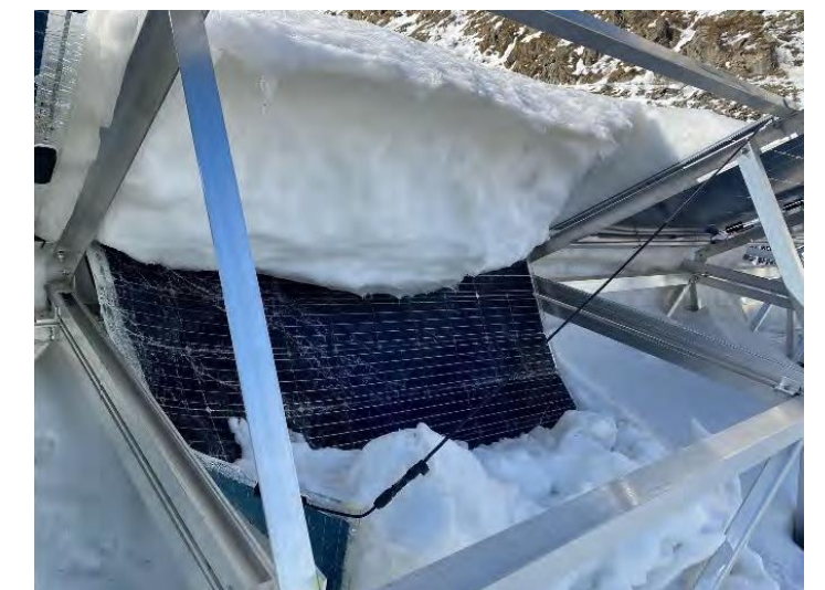
module tilting due to overload
