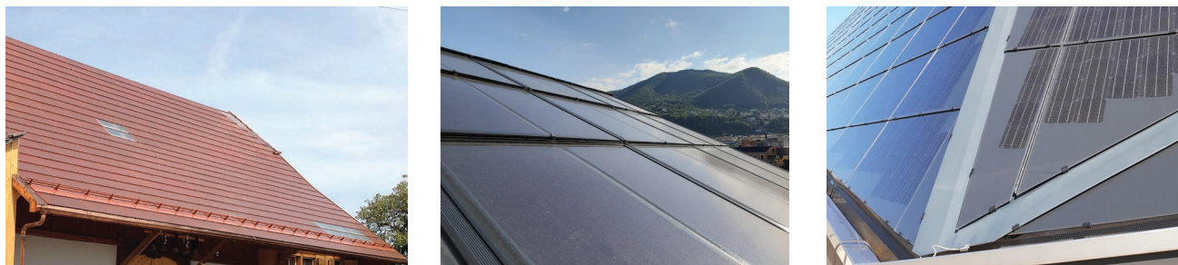
Figure 3.6 Left: Renovation featuring terracotta BIPV roof tiles on a historic farm in Ecuwillens, Canton of Fribourg, Switzerland; middle: solar shingles in a discontinuous roof; right: special roof parts for the Umwelt Arena in Spreitenbach, Switzerland. The modules are in an “all black” appearance with a black backsheet and covered interconnectors between the cell strings. Architect: Rene Schmid. Photos courtesy of Patrick Heinstejn, CSEM (left) SUPSI; Flisom-Schweizer (middle); P. Bonomo (right).
