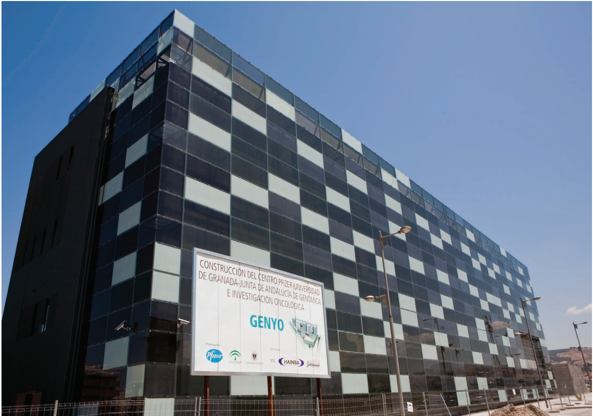
Figure 5.96 Pedestrian view of the Genyo Research facility, showing the BIPV south and west façades under construction. Credits: Onyx Solar.
