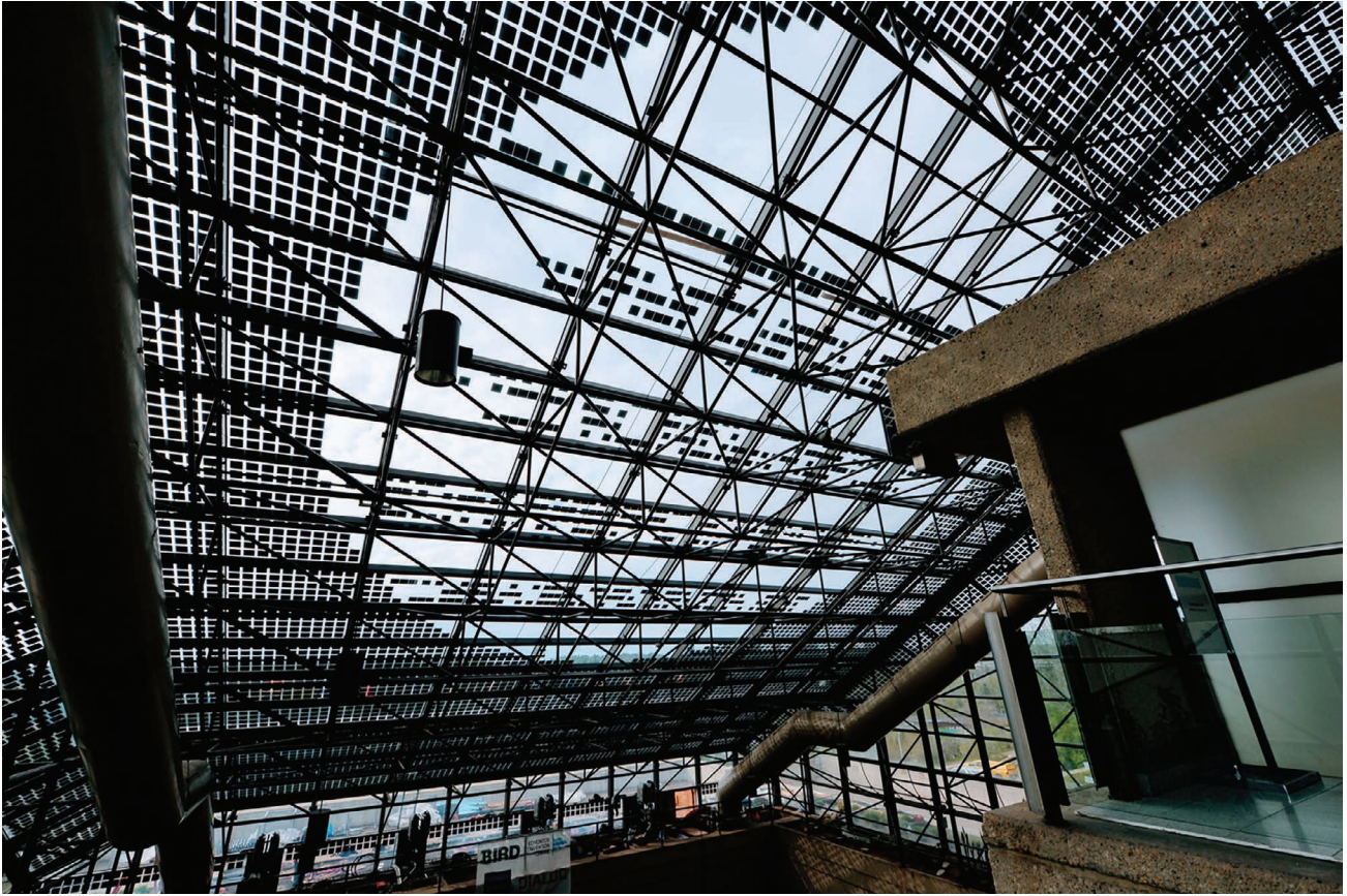
Figure 5.57 Skylight oculus at Edmonton Convention Centre. Credits: Onyx Solar.
