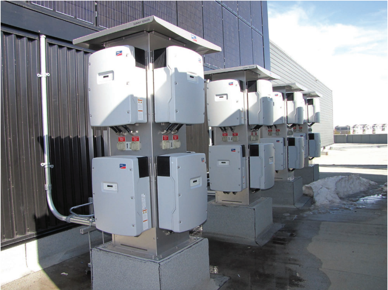
Figure 5.70 Rooftop string inverters at Jeanne & Peter Loughheed Performing Arts Centre. Credits: Credits: Gordon Howell, HME.
