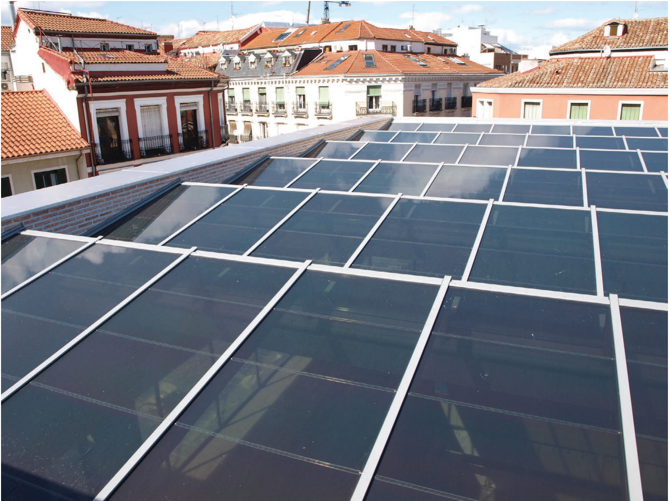
Figure 5.45 Exterior view of the BIPV skylight at San Antón Market. Credits: Onyx Solar.
