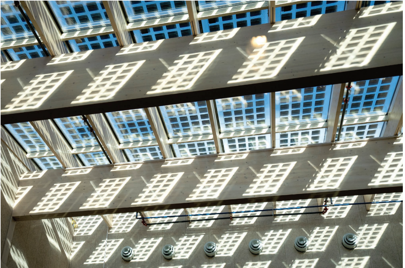
Figure 3.9 BIPV skylight application using insulated glazing with lower cells density for daylight transmittance at the “house of choice” designed by White Architects in Stockholm.
