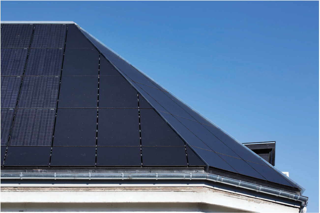
Figure 5.33 Close-up of the BIPV roof at Andreas Bjørns St.1. Credits: Dorte Krogh.
