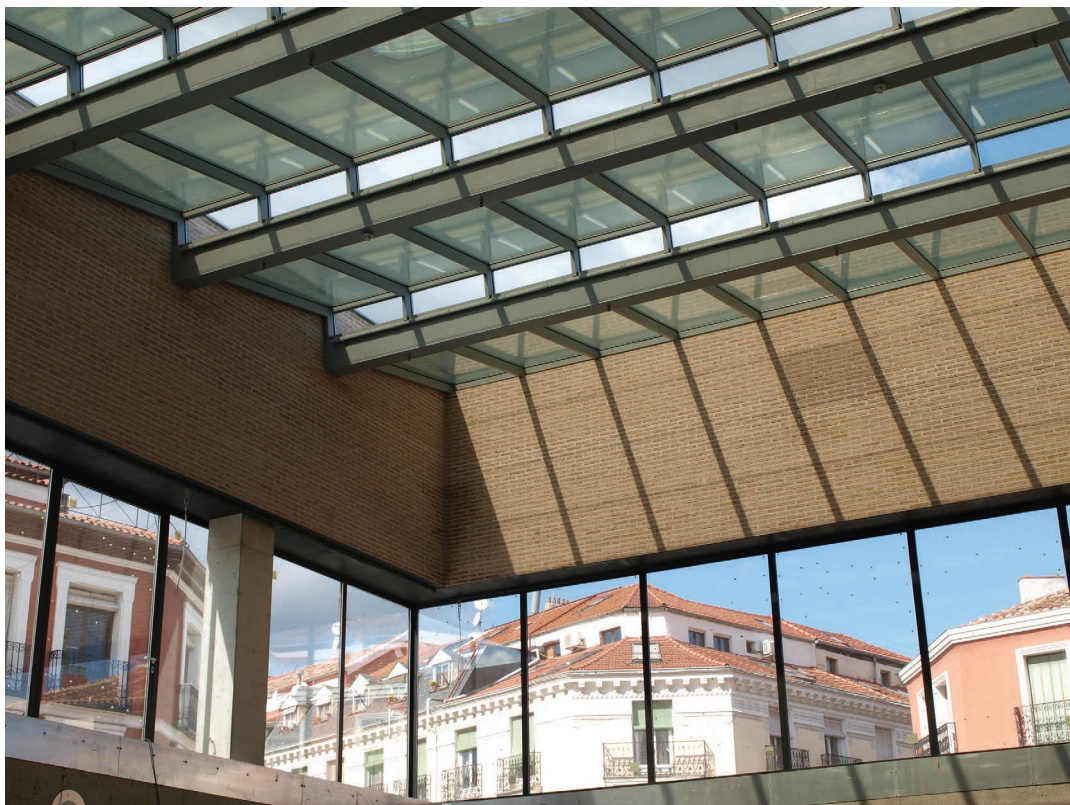
Figure 5.44 Interior view of the BIPV skylight at San Antón Market. Credits: Onyx Solar.
