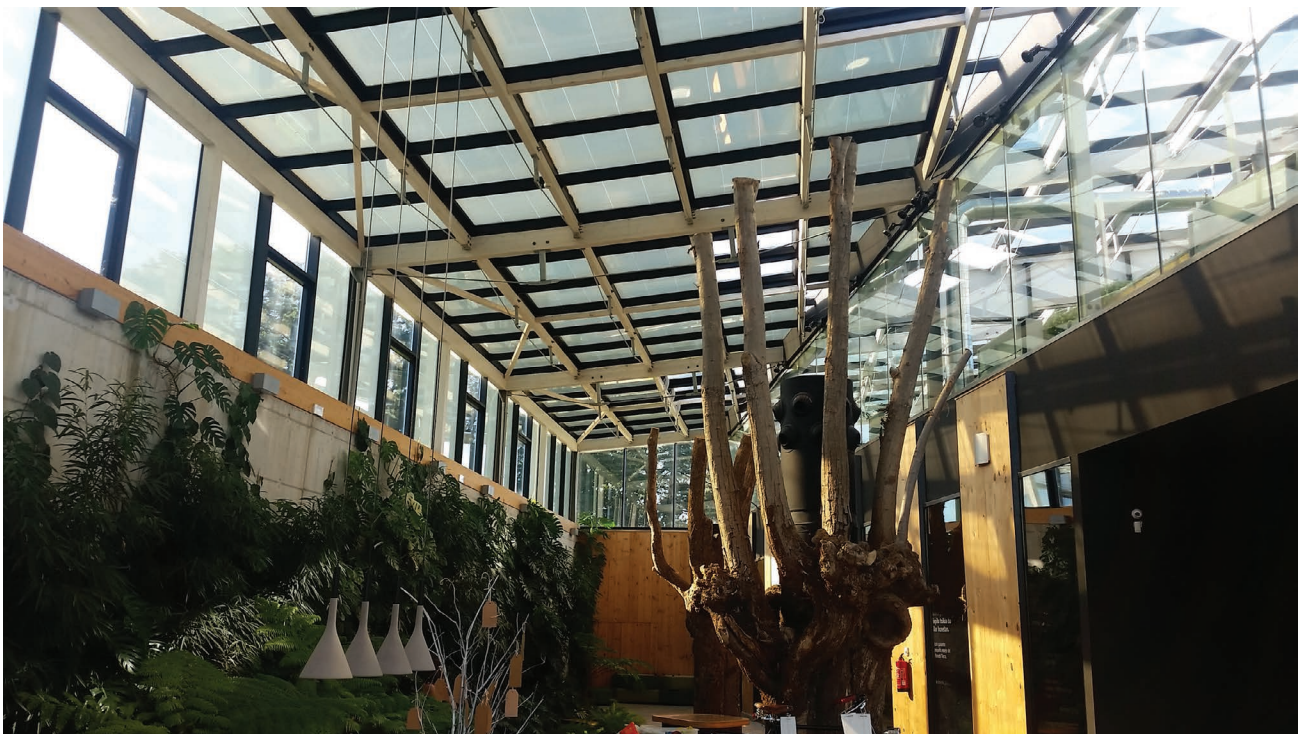
Figure 5.50 Interior view of BIPV curtain wall and skylight at the Azurmendi Restaurant. Credits: Onyx Solar.
