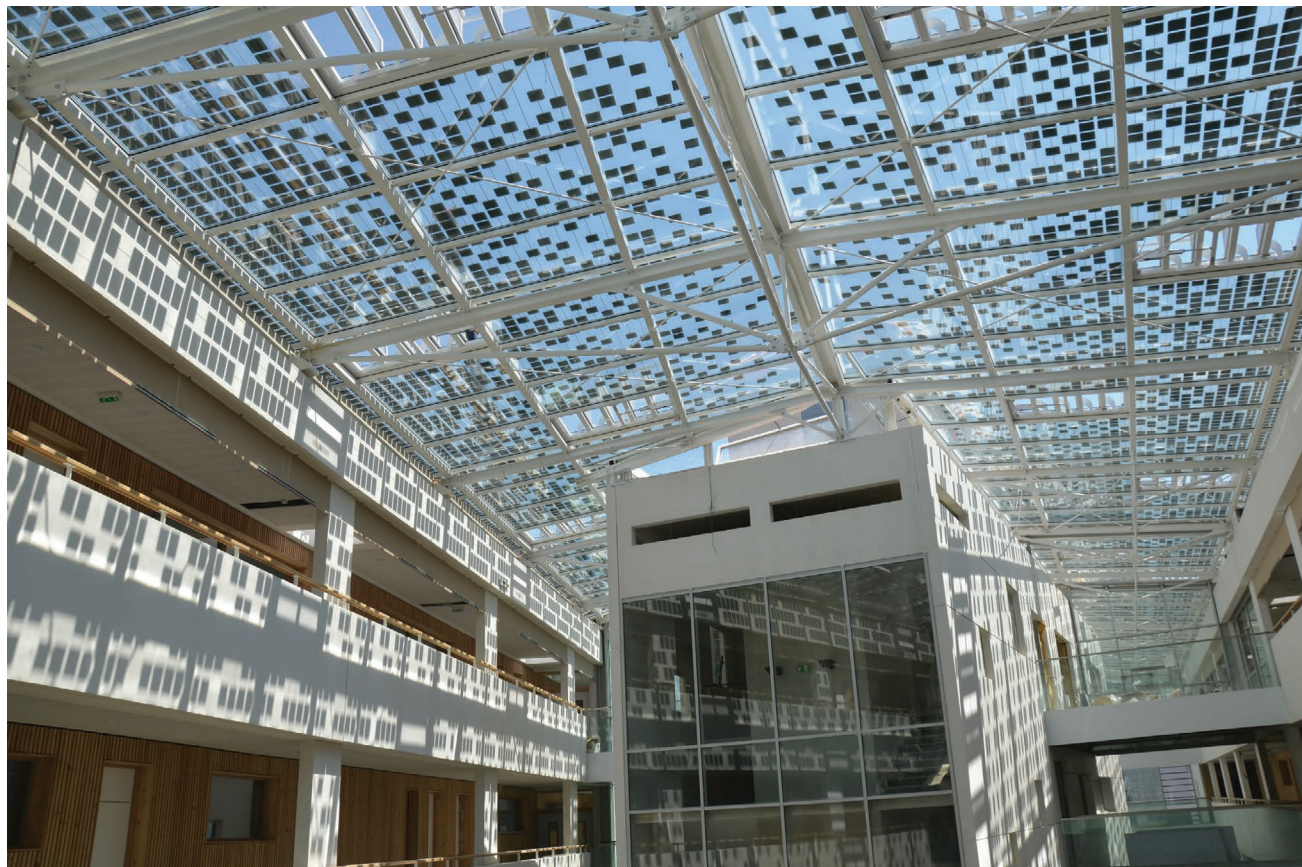
Figure 2.4 Semi-transparent BIPV skylight using c-Si solar cells at a school, in Courbevoie, France. Photo credits: MTECH & CSTB.
