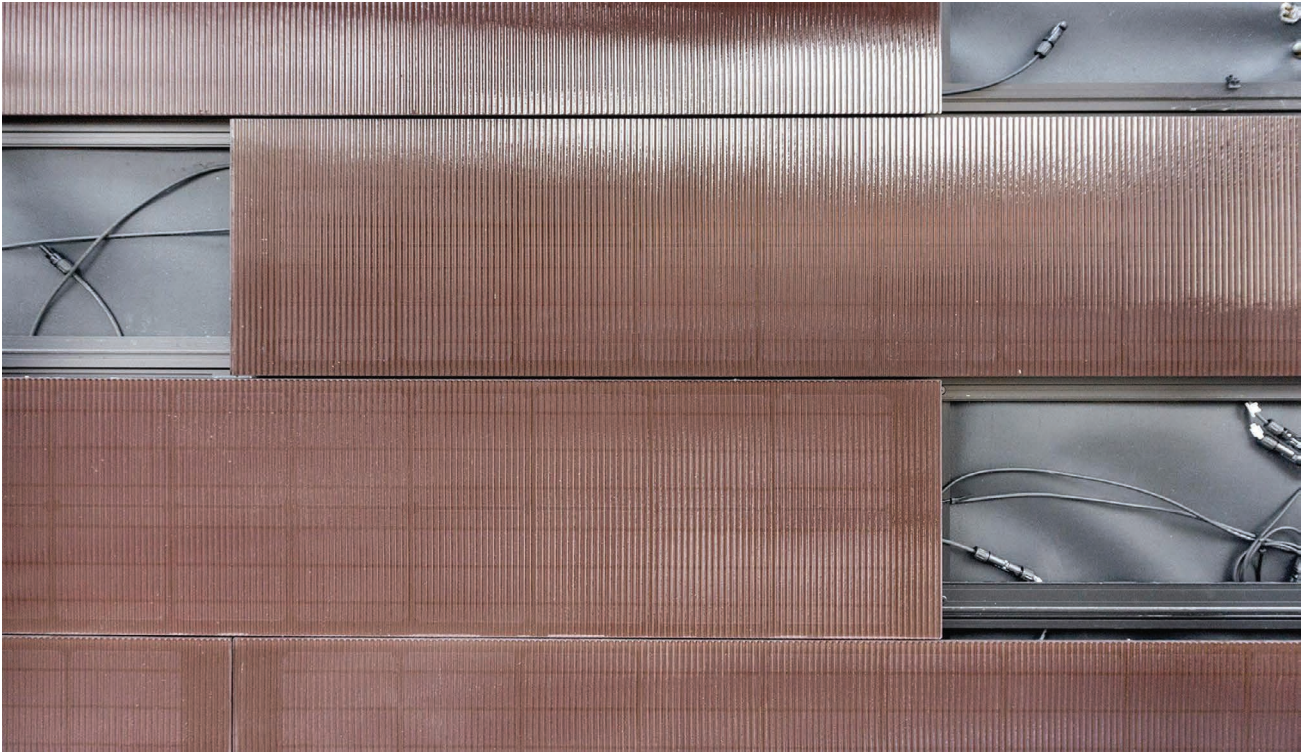
Figure 5.23 Detail of the BIPV façade at Solaris 416. Credits: Isa Zanetti, SUPSI.
