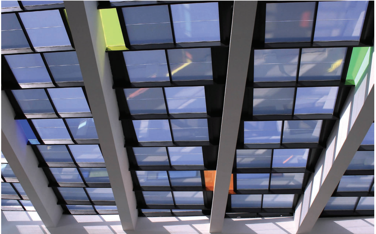
Figure 2.5 Retrofit of a skylight made of semi-transparent a-Si BIPV modules, in the historic Béjar Market in Salamanca, Spain. Photo credits: Onyx Solar.
