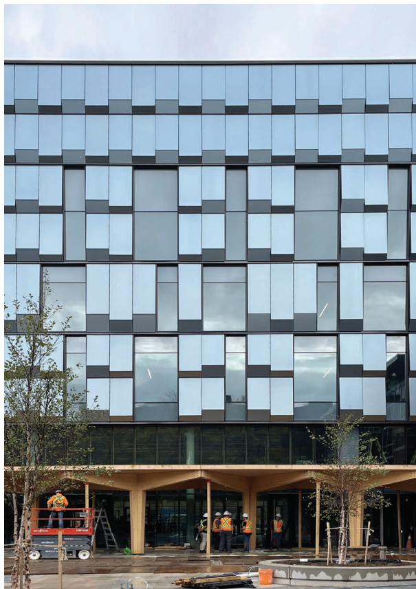
Figure 5.91 Close-up of the Fanshawe College Innovation Village BIPV rainscreen. Credits: Diamond Schmitt Architects.
