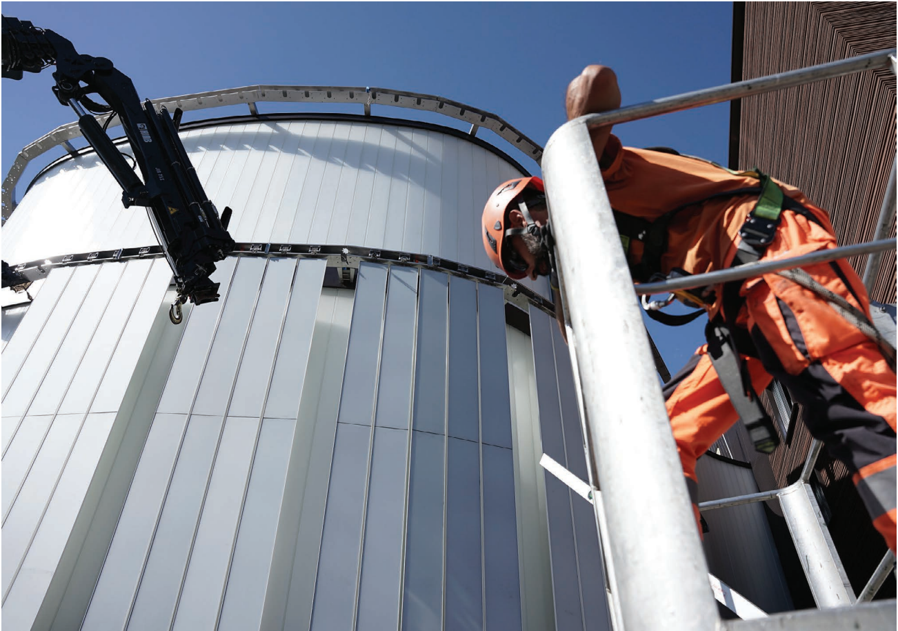
Figure 5.131 Installation of the white movable BIPV solar shading louvres. Credits: Franklin University.
