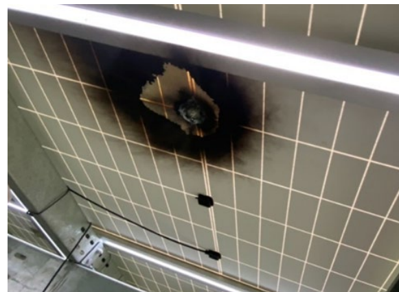
Figure 18: Module with burnt junction box resulting from unstable connection in the junction box.
