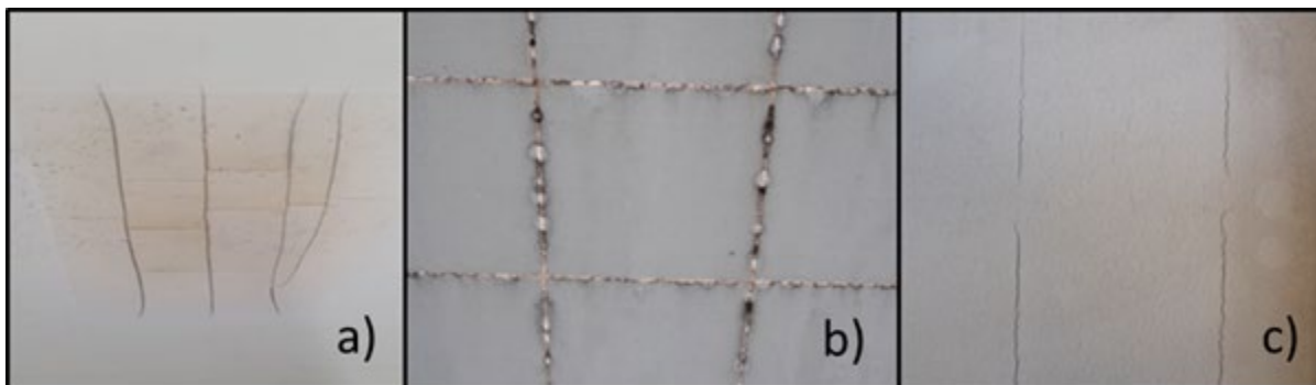
Figure 19: Backsheet crack types. a) cracked backsheet beneath a hot cell/temperature induced crack. b) squared cracks beneath cell interspaces; thermo-mechanical induced crack combined with photo-oxidative degradation. c) longitudinal cracks located beneath busbars; thermo-mechanical stress induced crack [69].
