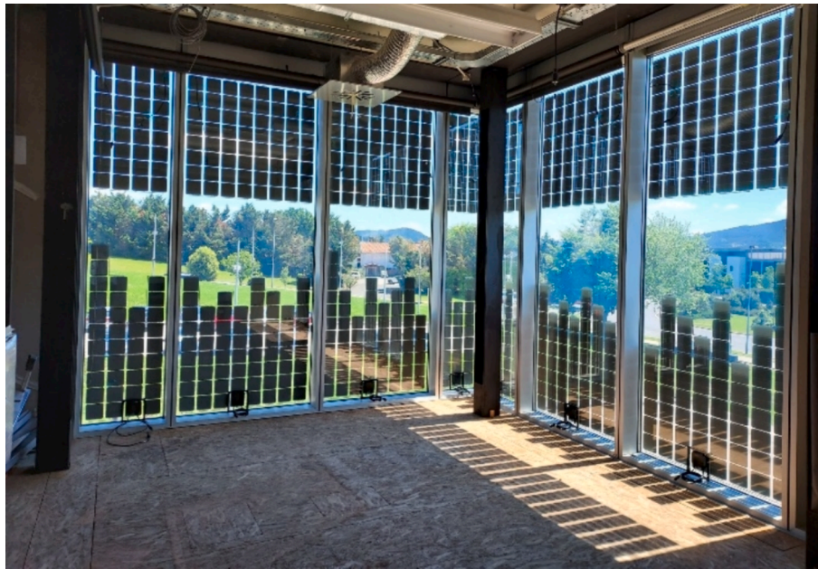
Fig. 1. PV semi-transparent glazing manufactured by Onyx Solar and installed in the Kubik experimental building at Tecnalia facilities in Derio, Spain, within the BIPVBoost project. Source: Eneko Setien, Tecnalia
