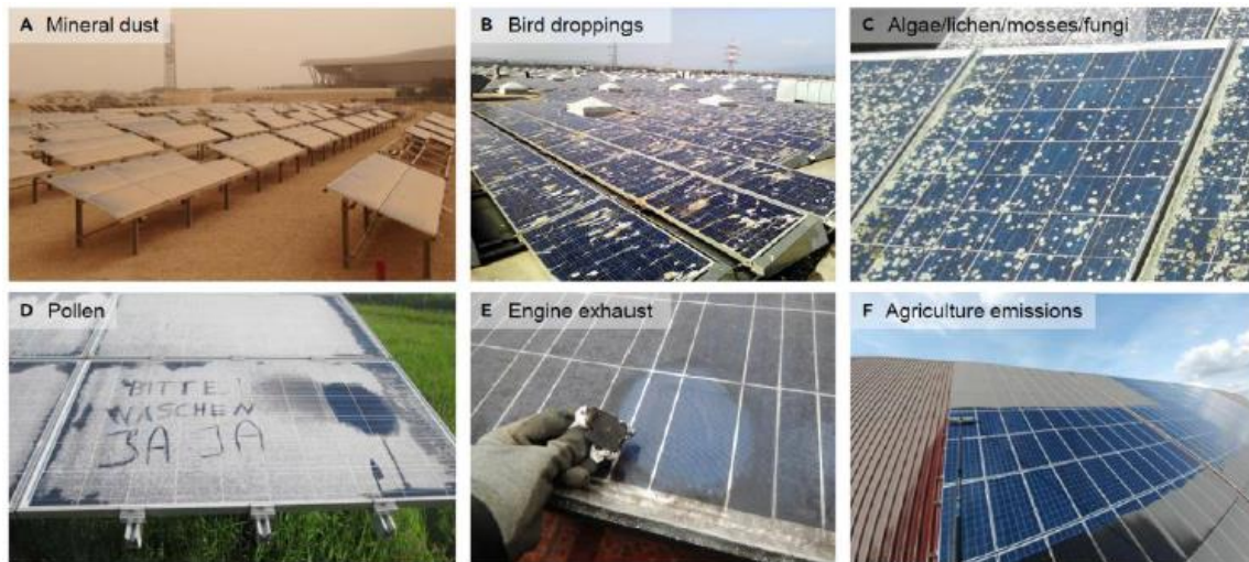
Figure 12: Examples of different sources of soiling buildup in PV arrays [152].
