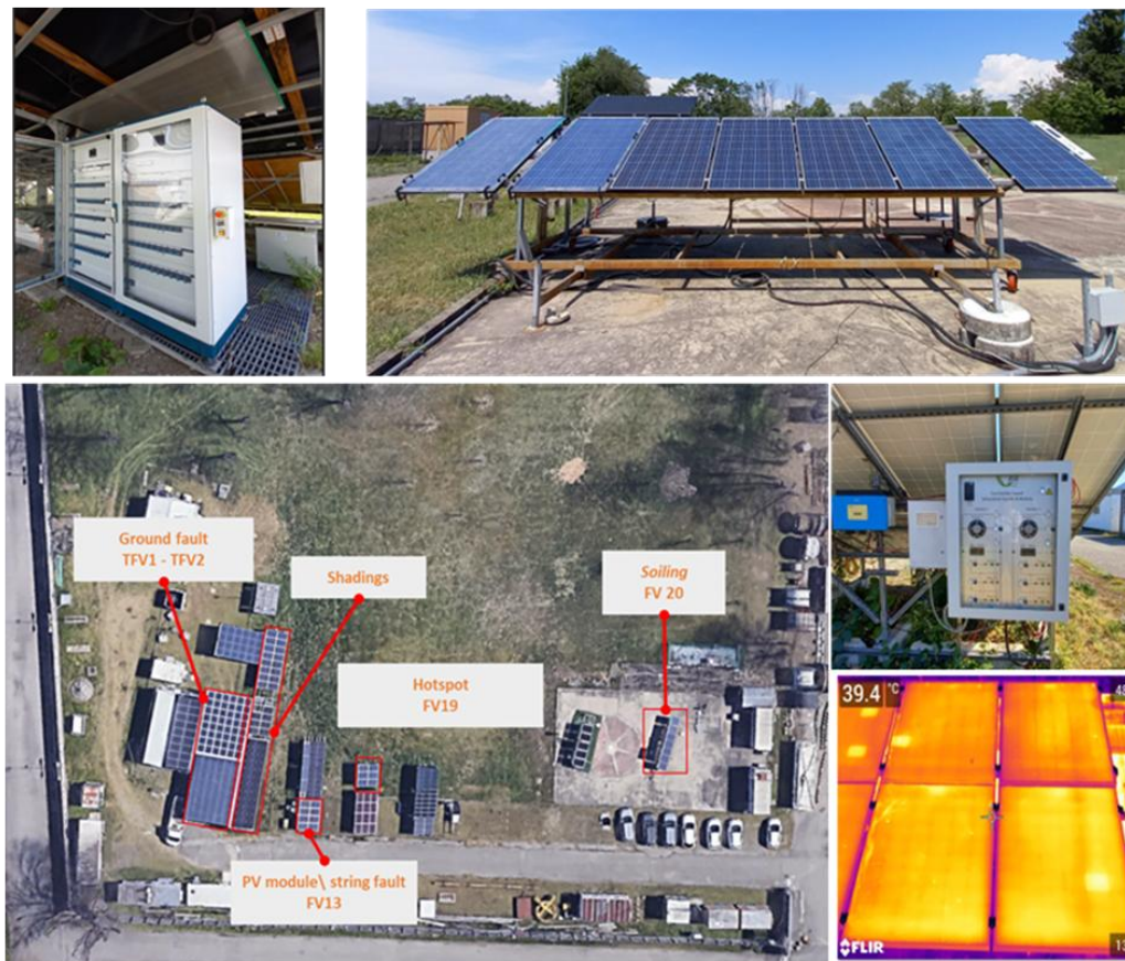
Facility Guasti FV
