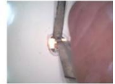
6. Separating bus bars
