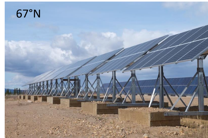
136 kW solar PV array in Colville Lake, Canada operated by the Northwest Territories Power Corporation
