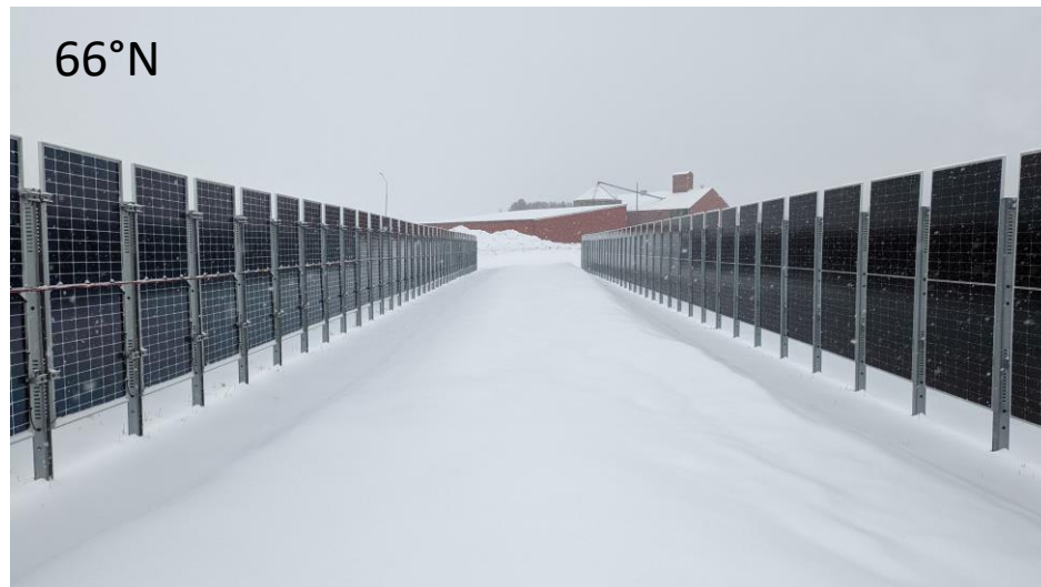
100 kW vertical bifacial PV pilot plant near Luleå, Sweden constructed by the Sunna Group
