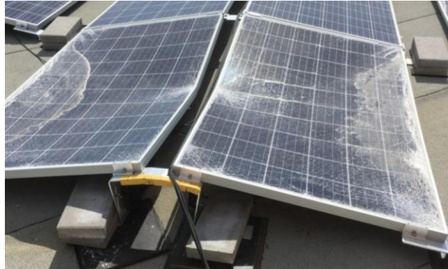
Damage due to snow loads and improper clearing. Images courtesy of Mattias Lindh, Alexander Granlund (RISE)
