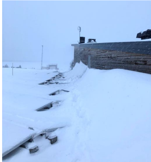
Rooftop PV (Piteå, SE)
