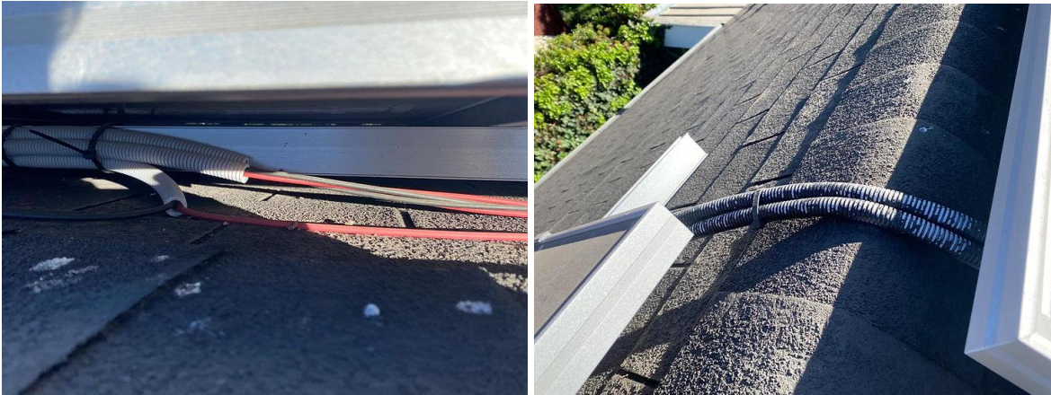
Figure 24: Solar cabling exposed directly to sunlight, compromising the whole project and even putting the property at risk. Incorrect use of conduit for transporting solar cables.
