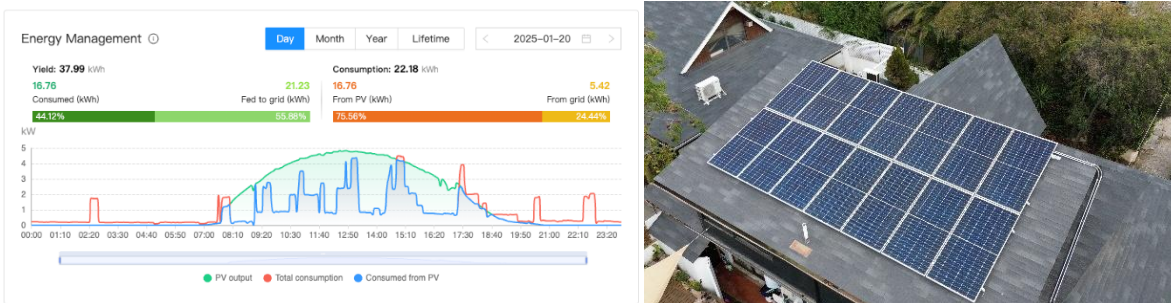
Figure 22: (left) Hourly monitoring of a rooftop installation; (right) the solar residential installation (Source: Solar Fotovoltaica Chile).
