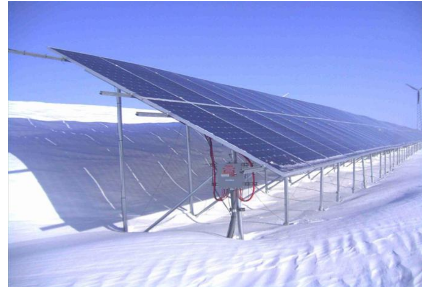
A row of PV modules in Kotzebue, Alaska, with an approximately 3-meter-high snow drift behind the row.
