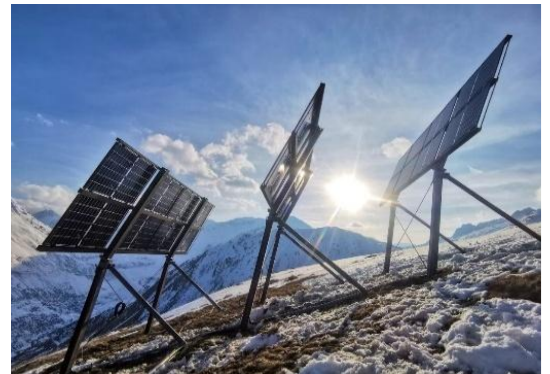
Photo credit: Sedrun Solar
