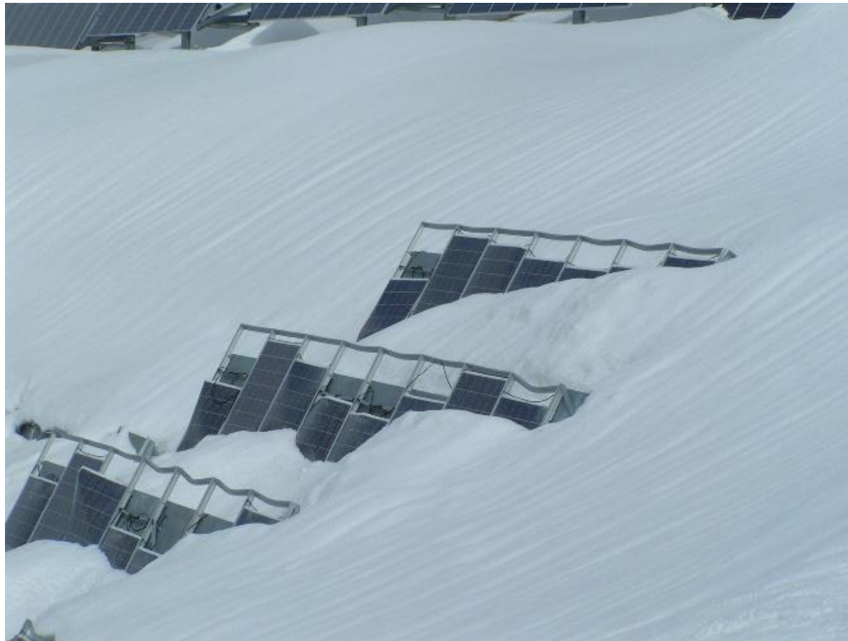
PV system at Wildkogel, Austria => Wrong site assessment
