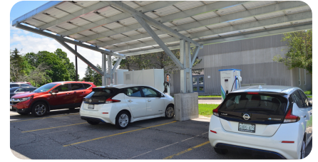
A PV-powered electric vehicle charging station.
