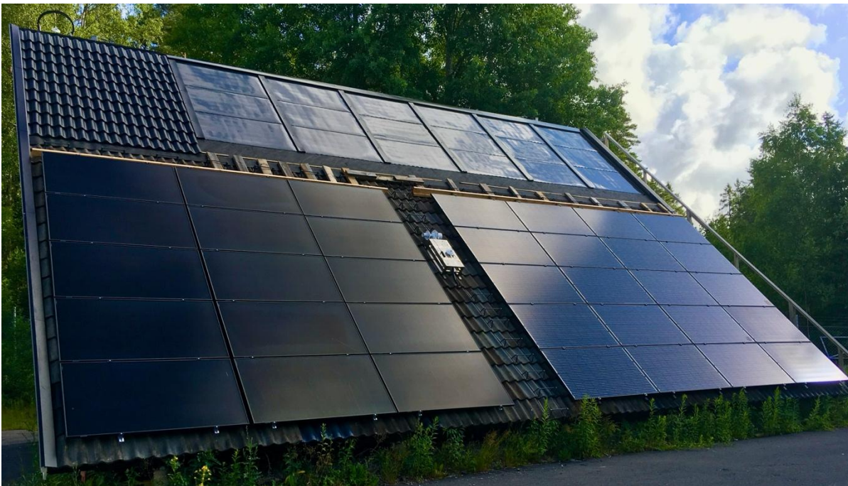
Figure 12: Close-up photo of PV arrays at RISE. The PV array connected to the battery system is in the lower right corner (Source: RISE).
