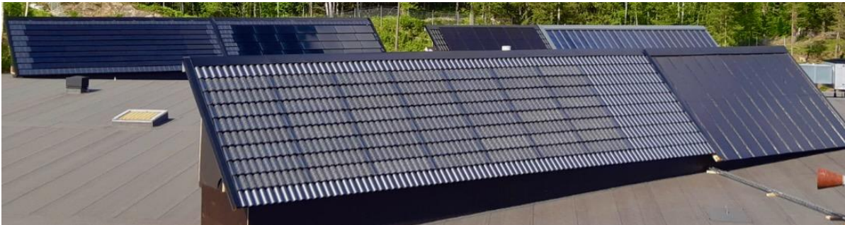
Figure 11: Overview of the PV array systems at RISE laboratory in Borås, Sweden (Source: RISE).
