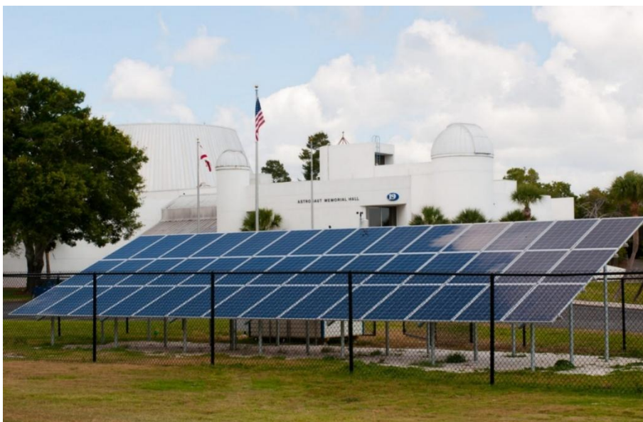
Figure 7: A PV + BESS installed in a school through the SunSmart E-shelters program (Source: UCF).
