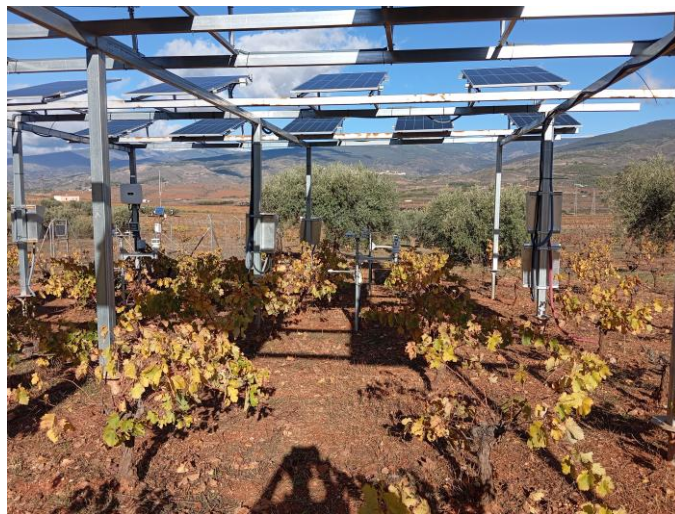
Figure 31: Corrosion visible on the structural elements of an elevated AV research installation after only one year of operation in Almería, Spain. (Photo credit: Álvaro Fernández Solas, DLR)
