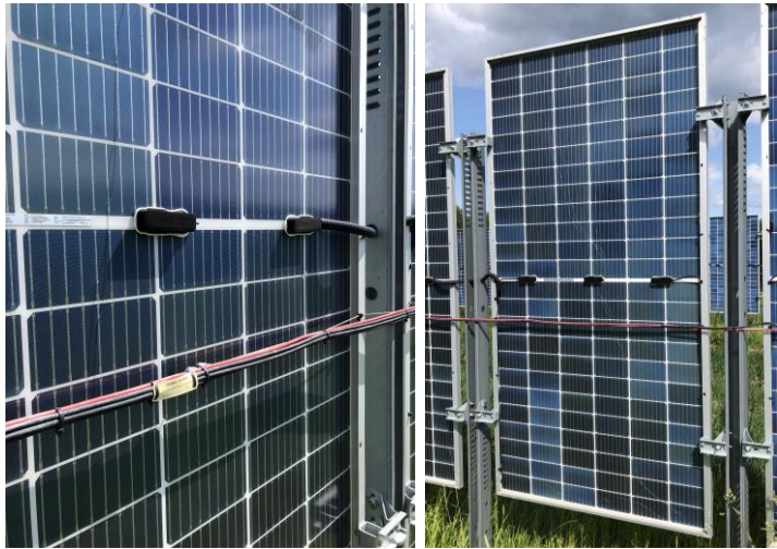
Figure 39. Connecting cables back to the inverter cause shading on the PV modules (left), and the PV module on the right has fractured glass, with the main fracture extending from the bottom-right corner to the top-left corner. (Photo credit: Pietro Elia Campana, Mälardalen University)
