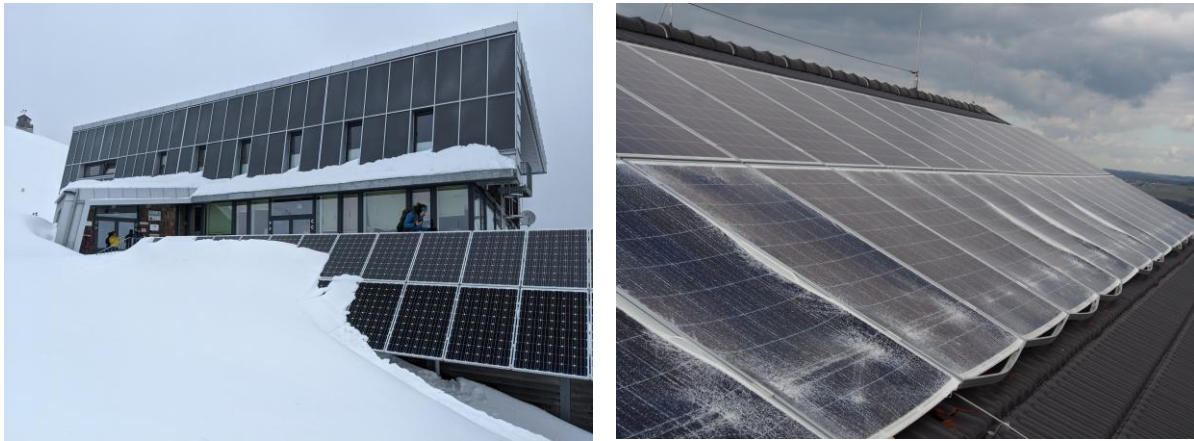
Figure 10: a) uneven snow load on a BIPV-installation, b) BAPV-system with broken modules and frames after a winter with heavy snow loads (Photo credit: Gabriele Eder/OFI).
